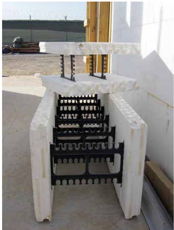
Similar to LEGO® building blocks, the ICFs snap together one on top of the other, with each segment adhered to the other with glue, to make a wall. (U.S. Air Force photo)
