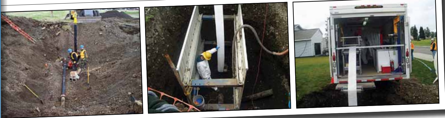
Replacing pipes using traditional (non-trenchless) methods requires 40-wide excavation (left). During pipe repair at JBER using trenchless technology, a flexible liner is impregnated with epoxy (right), then pulled into existing pipe (center). (U.S. Air Force photos)
