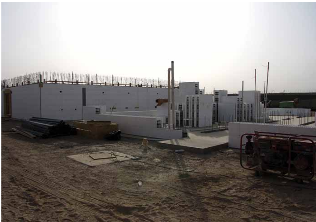
Because of their light weight and compactness, ICFs create a small construction footprint, making them ideal to use for tight construction sites. (U.S. Air Force photo)
