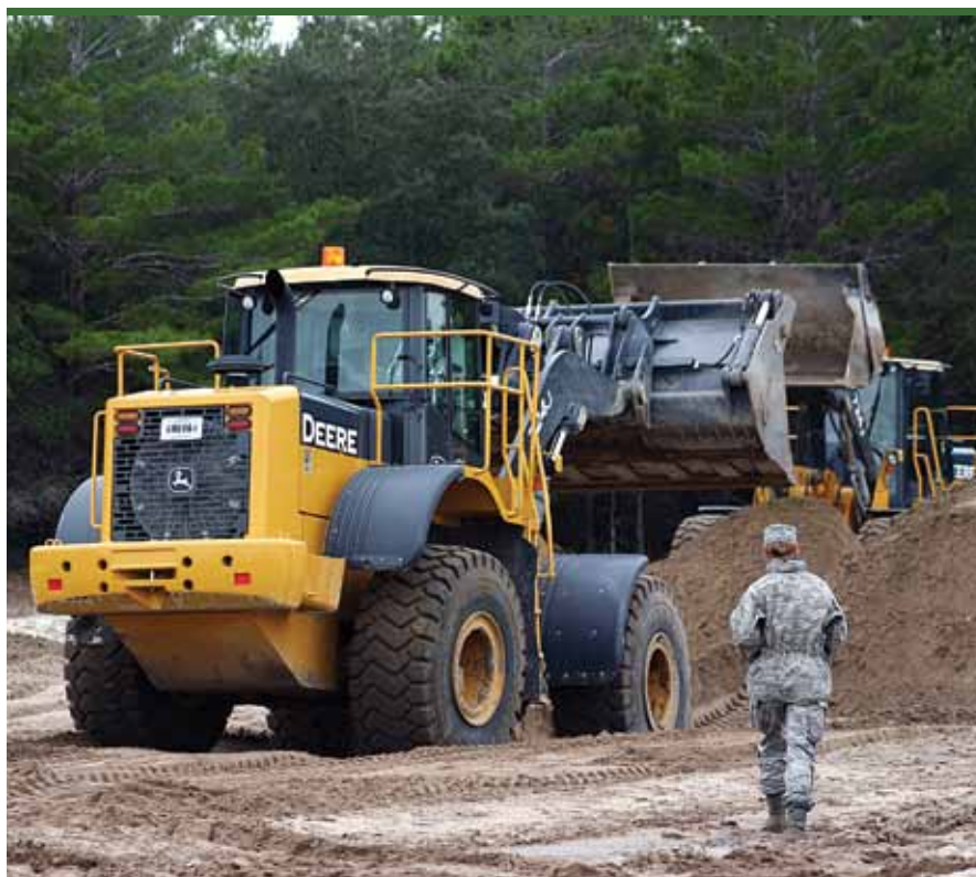
During the Officer Education Course (OFE) at the Silver Flag Exercise Site, Tyndall AFB, Fla., a second lieutenant learns how to utilize heavy equipment to construct an earthen berm containment system for POL bladders. All new civil engineer officers are required to take AFIT's WMGT 1010 (Air Force Civil Engineer Basic Course), which concludes with a week-long OFE course. (photo by Ms. Teresa Hood)
