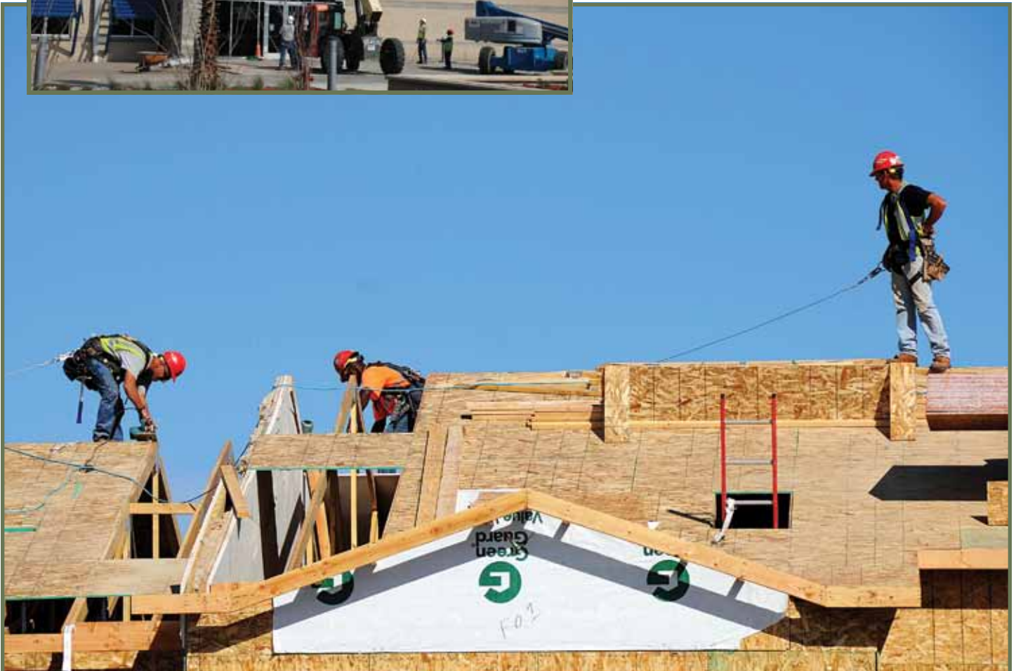
Photo below: Contractors from Fairbanks Roofing Company install a roof on one of the new housing units at Eielson AFB. AFCEE has managed the construction and renovation of 349 new units and 29 pre-existing units on Eielson AFB, Alaska. (photo by SSgt Tia Wilson)
