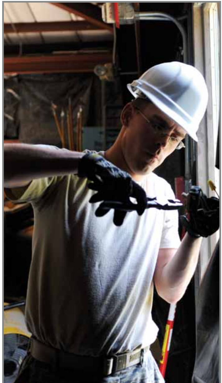
SrA Brandon Long, an electrician assigned to the 316 CES, re-routes a light switch during renovation of the Honor Guard building at Joint Base Andrews Naval Air Facility, Md. (photo by SSgt Renae Saylock)
