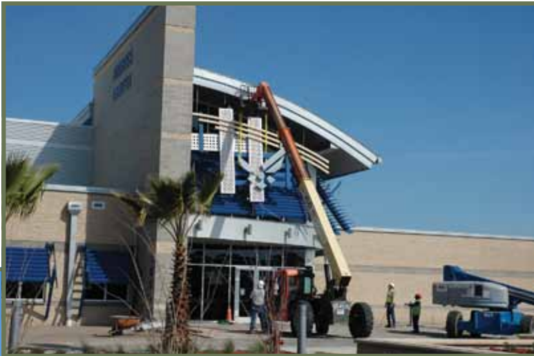
Photo left: Work nears completion on the new fitness center at Tyndall AFB, Fla. The fitness center will be the Air Force's first building to meet the U.S. Green Building Council's Leadership in Energy and Environmental Design Platinum level. (photo by Mr. Michael Hopper)
