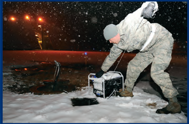
SSgt Matthew Nelson, 35th CES, starts a water pump to get water out of the steam lines that collected as a result of power loss from the earthquake. (photo by SSgt April Quintanilla)
