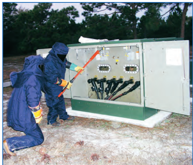
AFIT's recent satellite seminar on electrical safety program management was an opportunity for Air Force electrical experts to emphasize the use of proper techniques and equipment to safely perform tasks such as the operation of an above-ground medium-voltage switch. (U.S. Air Force photo)
