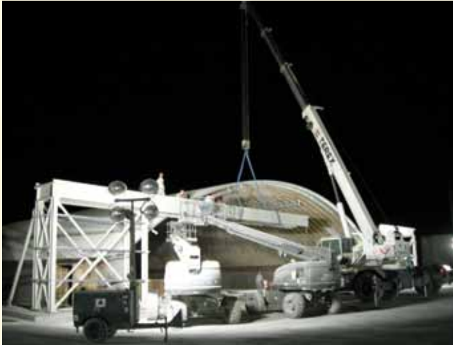
RED HORSE Airmen erecting a 120 foot wide aircraft hangar door on one of the Super K-Spans. (photo by CMSgt Jay Campbell)
