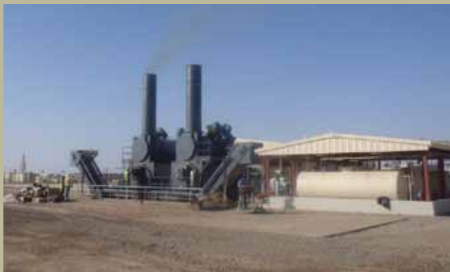
Two incinerators constructed at Camp Leatherneck, Afghanistan, in January, can operate around the clock and burn up to 12 tons of solid waste each per day. The four more incinerators are planned for the camp will bring the capacity to 88 tons per day. (U.S. Air Force photo)
