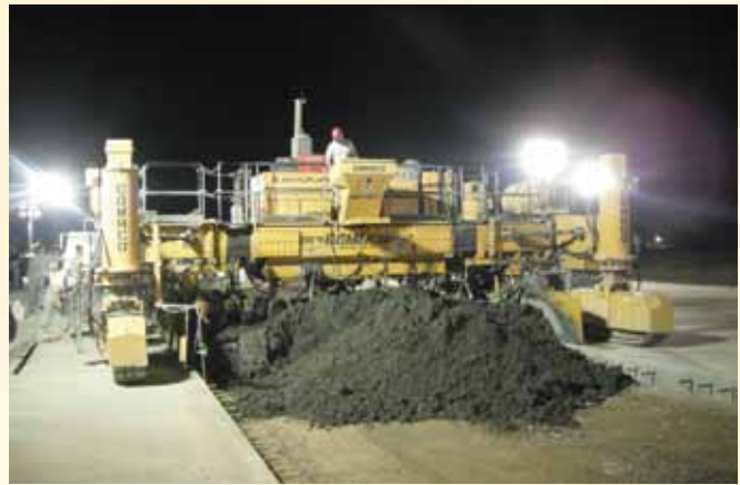
RED HORSE Airmen worked day and night constructing Dwyer's paved runway. Slip-form paving equipment eliminated the need for formwork. (photo by CMSgt Jay Campbell)
