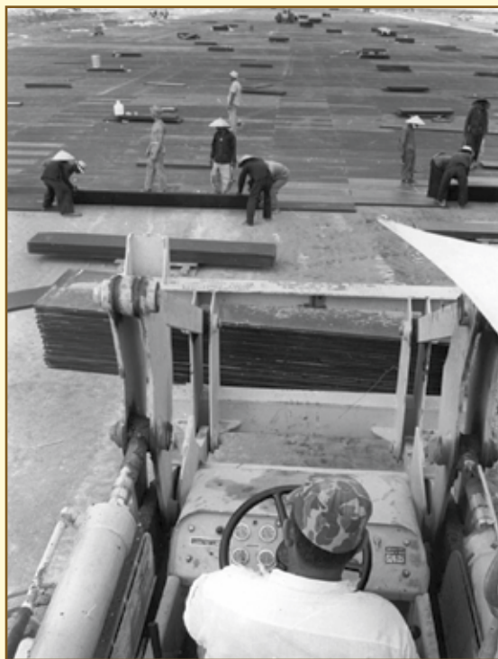
Workers lay AM-2 matting for Tuy Hoa's 9,000 ft runway. (U.S. Air Force photo)
