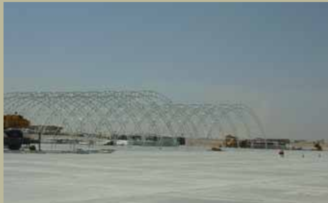
Part of the $700M construction project at Camp Bastion includes the shelters whose contractor-built frames are shown here. (U.S. Air Force photo)
