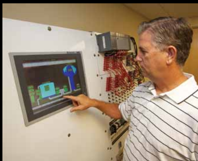
Mr. Dennis Hatcher, a CEMIRT ICS technician, uses a systems operator screen to test an ICS program developed at CEMIRT, HQ AFCESA, Tyndall AFB, Fla. (photo by Mr. Eddie Green)
