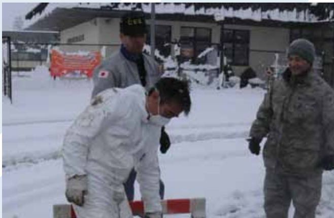
Members of 35 CES heating, ventilation and air conditioning shop prepare to go underground to repair a steam line broken by the earthquake and tsunamis. (photo by SSgt Rachel Martinez)
