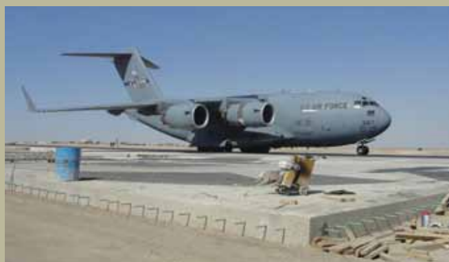
This newly completed strategic airlift apron is part of phase one of a $700M airfield construction program taking place at Camp Bastion in Afghanistan. (photo by Maj Patrick Suermann)
