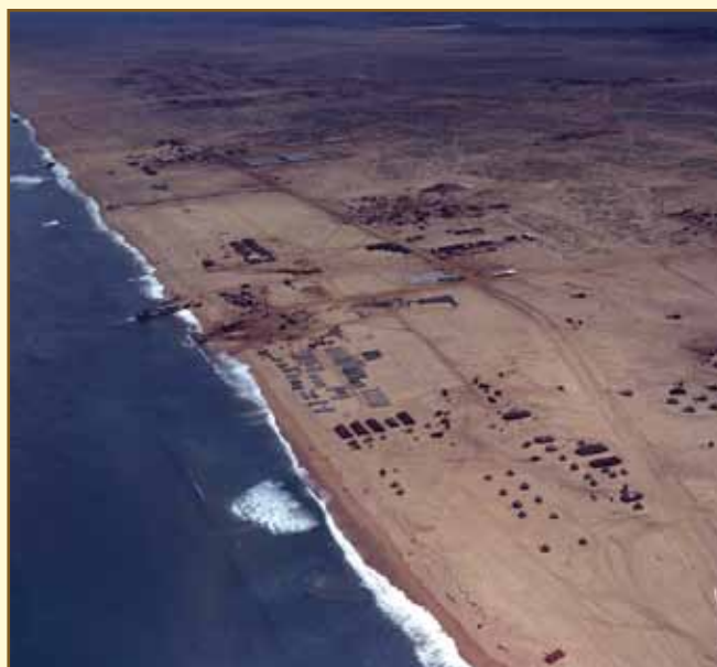
An aerial view of the base under construction at Tuy Hoa, directly on the South China Sea. (U.S. Air Force photo)
