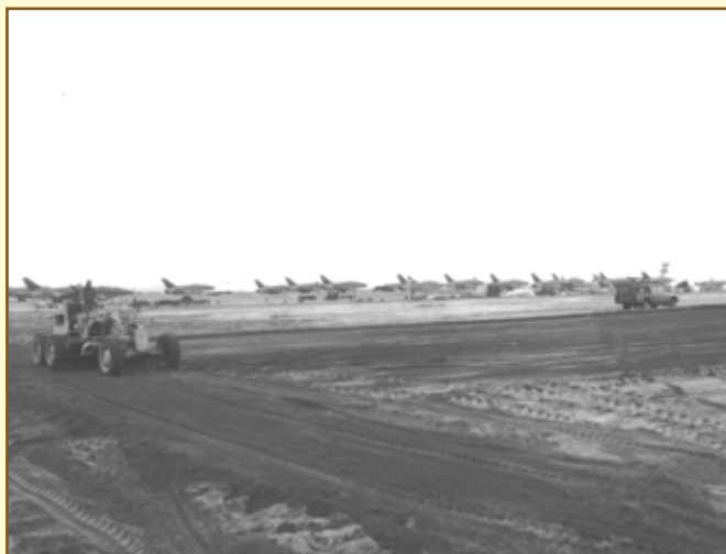
820th Civil Engineer Squadron (HR) members prepare a site for construction of a maintenance apron at Tuy Hoa AB with F-100s parked in the background. (U.S. Air Force photo)
