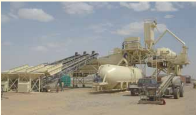
A state-of-the-art concrete batch plant shipped to Afghanistan for Dwyer's construction. Once operational, the concrete batch plant produced twice as much concrete as three contractor-run plants at Camp Dwyer. (photo by CMSgt Jay Campbell)
