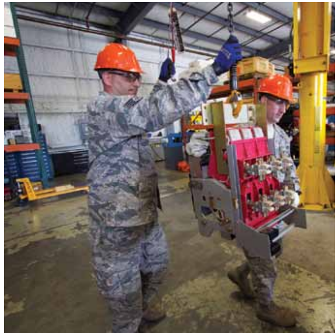
SSgt Justin Swanberg and TSgt Ernest Crook move one of Thule's newly retrofitted low-voltage circuit breakers for testing . (Photo by Mr. Eddie Green)
