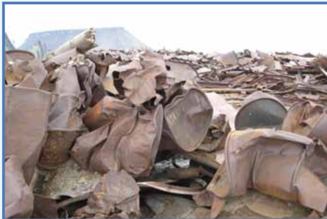
As part of a recycling project, the first shipment from Thule of scrap metal from deconstructed fuel tanks and other demolition netted the base more than $1M for reinvestment in environmental remediation projects. (photo by Mr. Todd DeGarmo)
