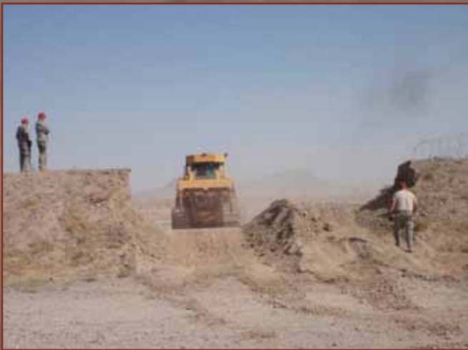
Using a Cat D7 dozer, CEs break through a berm (formerly the FOB perimeter) to access the project site and begin construction.
