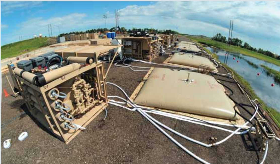
The ROWPU "plant" at Minot included eight 1,500 GPH ROWPUs and six bladders and from July 1-20, produced more than 3.9 million gallons of usable water. (photo by SrA Jesse Lopez)
