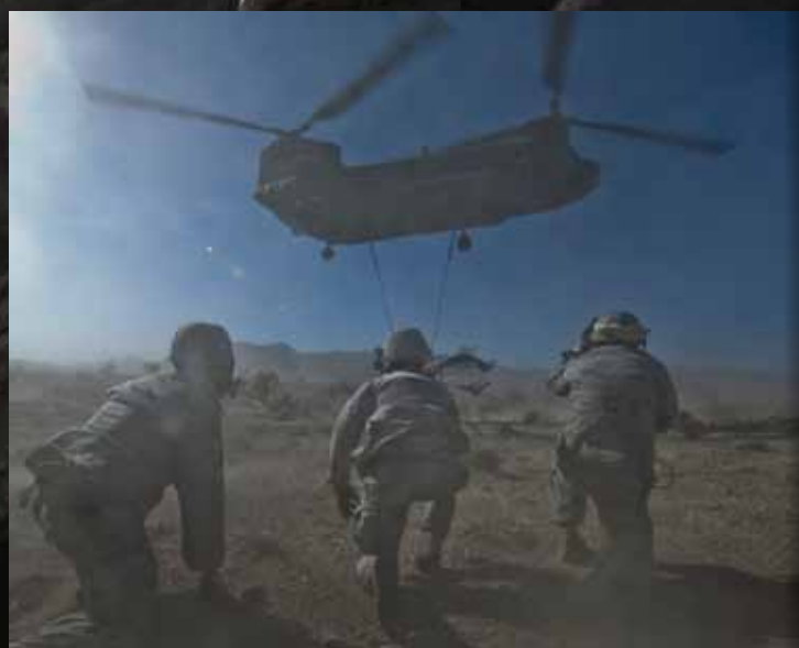
During cleanup of an F-15C crash site in southern Nevada, SSgt Ian Zerby, 820 RHS Airborne Flight, prepares to rig a CONEX box for sling load by a NG CH-47 Chinook and (inset) Airmen from the 820 RHS Airborne Flight take a knee as the Chinook recovers an aircraft part. (photos by A1C Daniel Hughes)
