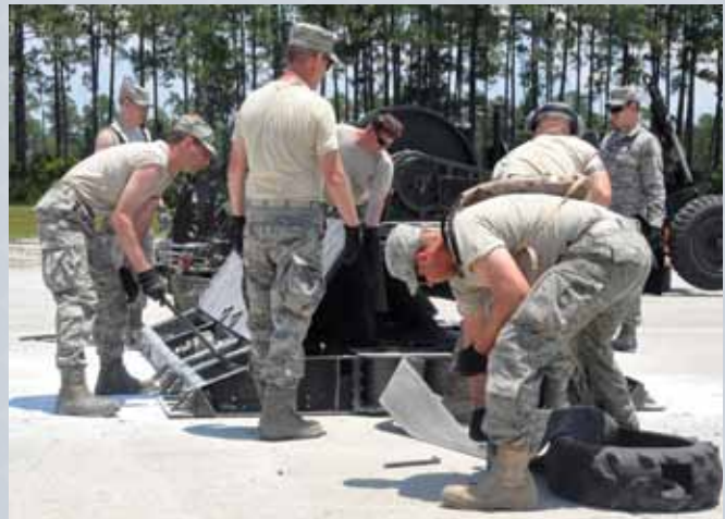
Power Production Airmen break down a mobile runway edge sheeve as part of a Silver Flag training exercise designed to improve their readiness capability. (photo by SSgt Grant Saylor)
