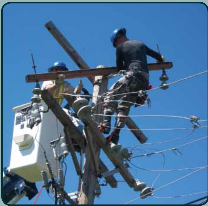
TSgt Phillip Wilson (left) and SSgt Austin Hollingshead, 375 CES, Scott AFB, Ill., repair a power pole at Little Rock AFB, Ark., after a tornado struck the base in April. (Courtesy photo)
