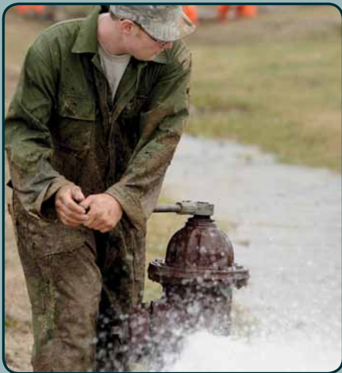
SSgt Justin England, 509 CES, flushes a repaired water main at Whiteman AFB, Mo. (photo by SrA Kenny Holston)
