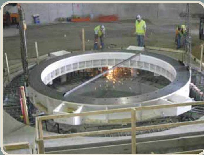
Construction of the 711th Human Performance Wing's centrifuge at Wright-Patterson AFB, Ohio. (U.S. Air Force photo)
