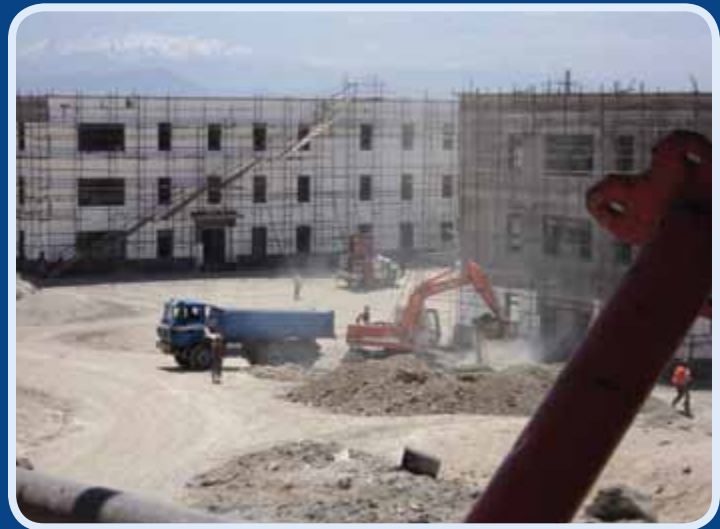
A construction team builds the National Defense University in Afghanistan, one of many projects managed by the AFCEE Contingency Construction Division. (courtesy photo)
