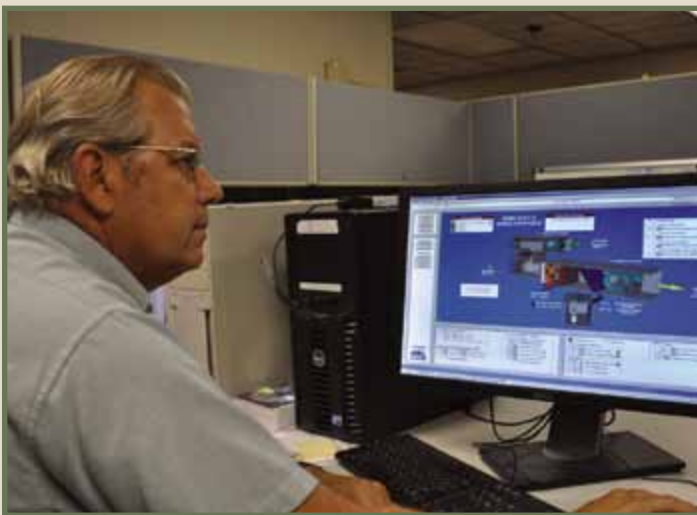
Mr. Michael Miller, 92 CES, Fairchild AFB, Wash., evaluates one of the base's three energy management control systems. (photo by Mr. Scott King)
