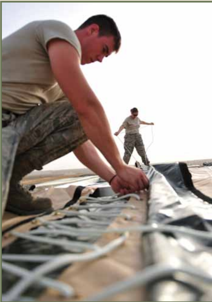
Members of the 380 ECES assemble a California medium shelter system, or CAMSS. (photo by SSgt Patrick Mitchell)
