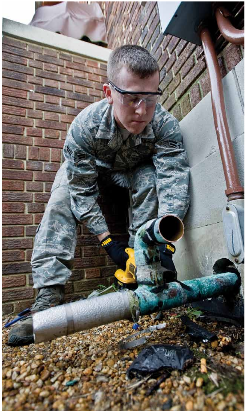
A1C William Davey, an HVAC apprentice with the 633 CES, replaces a water line for a chiller at JB Eustis-Langley, Va. (photo by SrA Stephanie Rubi)
