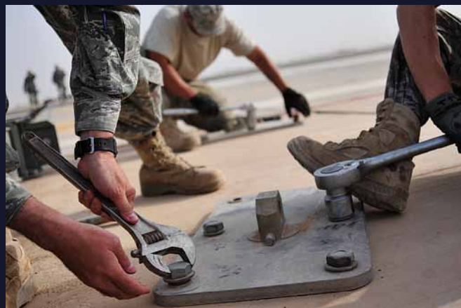
Power production craftsmen from the 332 ECES at JB Balad disassemble the anchor plates of a mobile aircraft arresting system on Oct. 15, 2011 to ready the base for transition to the Iraqi government. (Photo by MSgt Cecilio Ricardo)
