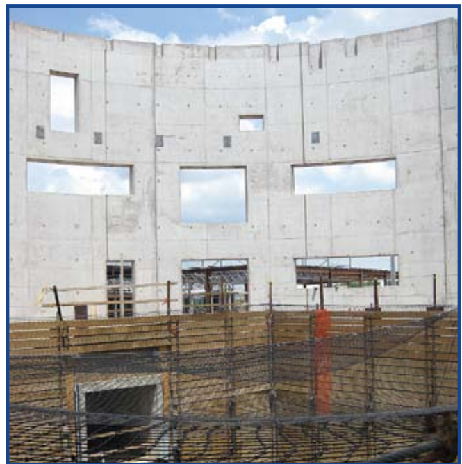
The retaining wall system of the future Air Force Centrifuge hall is composed of H-piles and underpinning, the utility access tunnel, and foundation pit personnel net, which is a safety feature to prevent construction workers from inadvertently falling into the 25-foot deep excavation. (photo by Mr. Kevin Hill)
