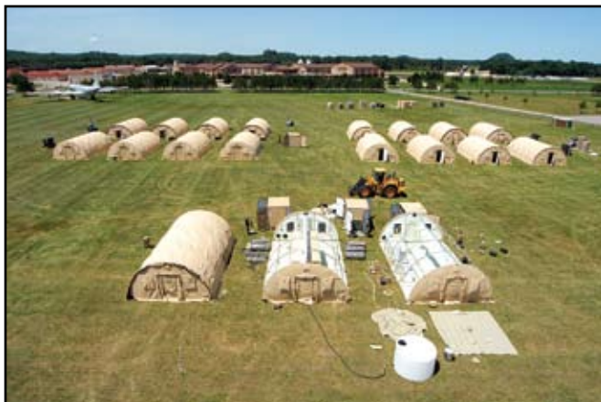
Assembly of tents for a Disaster Relief Beddown Set is almost complete at Volk Field, Wis. The tents were erected by members of the Kentucky Air Guard's 123rd Civil Engineer Squadron in about 14 hours as part of PATRIOT '09. (photo by A1C Max Rechel).
