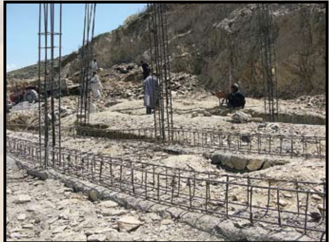
During quality assurance trips to remote sites, the Paktya PRT engineers often encountered construction challenges that required “do-overs” by the contractors, such as rebar constructed on unlevel foundation. (photo by author)
