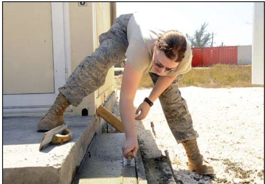
SrA Samantha Orem of the 142 CES floats concrete for a stair step during the squadron's participation in Exercise Tropical Hammer in Kingston, Jamaica. (photo by author)
