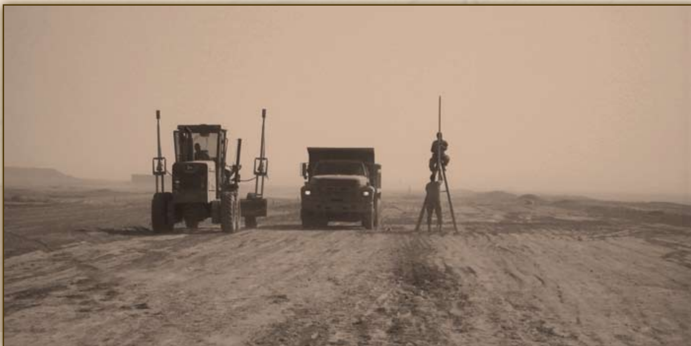
A1C David M. Smith secures a ladder for SrA Joseph Van Berkum as they stabilize the laser grading receiver. (photo by MSgt Gerald D. Haight)
