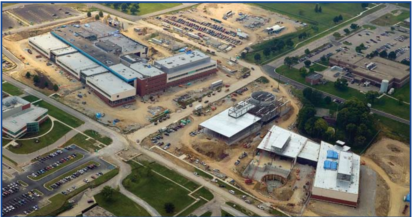
Southwest aerial view of the HPW construction through August 2009. (photo courtesy of Metroflyer, LLC)
