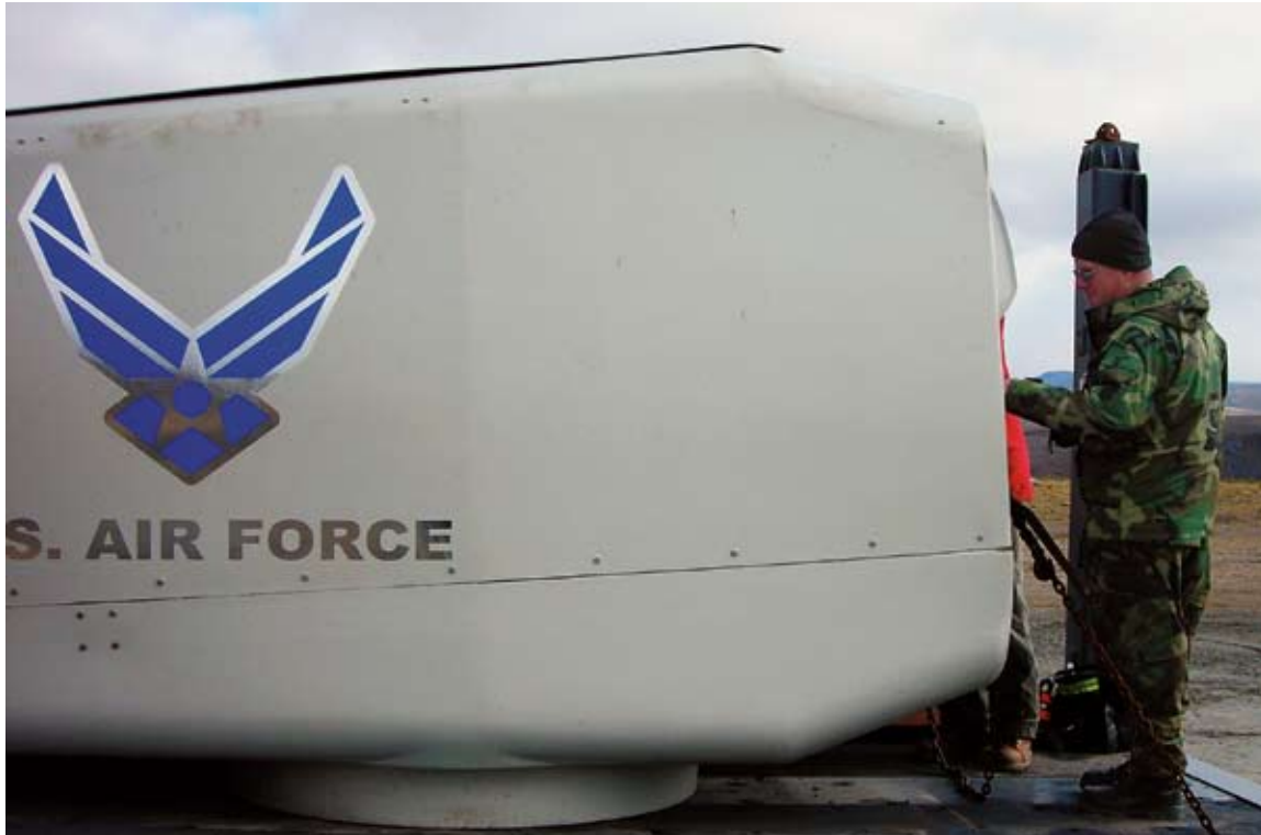
Far left: The completed wind turbine assembly. Left: MSgt James Fraser, 611 CES quality assurance NCOIC, inspects the turbine nacelle before its installation. (U.S. Air Force photos)
