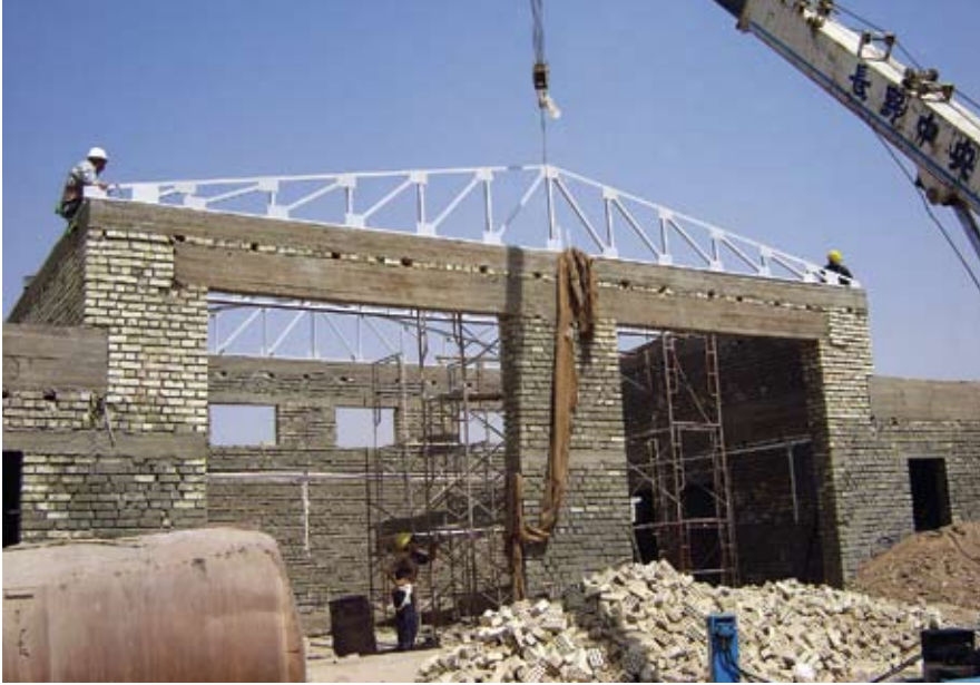
Iraqi workers place trusses on a firehouse, part of an AFCEE contract to rebuild the Iraqi infrastructure. (U.S. Air Force photo)
