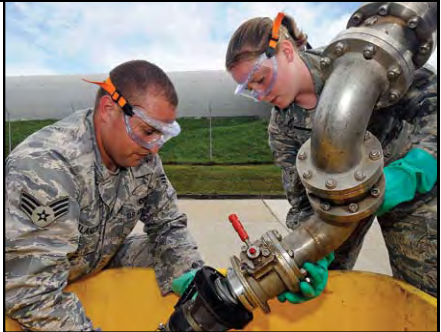
SrA Ivan Alandzak and A1C Jennea Allen, 52 CES, replace a single point nozzle over a drip-pan on one of Spangdahlem AB truck refueling stands. (photo by SrA Benjamin Wilson)
