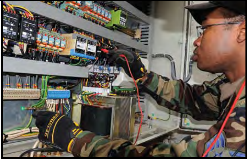
SSgt Taraus Boyd, 100 CES electrical technician craftsman, checks for proper voltage using a multimeter during troubleshooting procedures at the waste plant, RAF Mildenhall, England. (photo by SSgt Jerry Fleshman)
