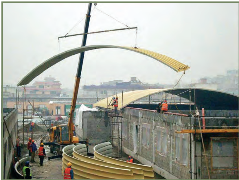
Photo left: The new Afghanistan National Army compound under construction in Kabul. AFCEE is managing the $18.3M project. (U.S. Air Force photo)
