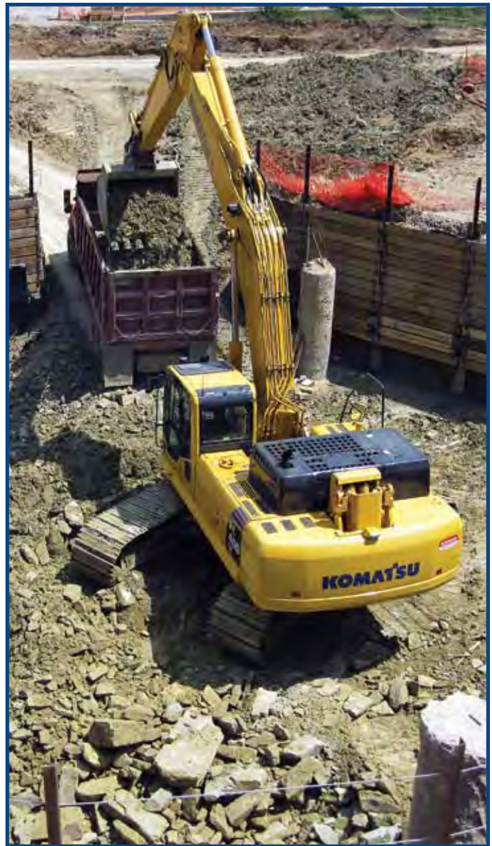
An excavator loads up a truck during excavation to build the foundation for the Disorientation Research Device facility at the Human Performance Wing, Wright-Patterson AFB, Ohio. (photo by Mr. Kevin Hill)
