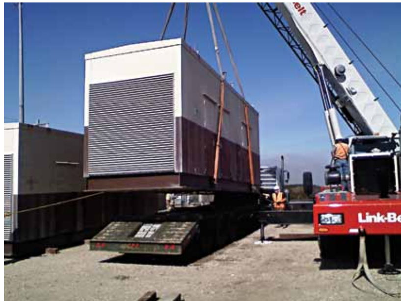
Experts from CEMIRT, Travis AFB, Calif., install a CEMIRT Emergency Power System, or CEPS, at Vandenberg AFB, Calif. (U.S. Air Force photo)
