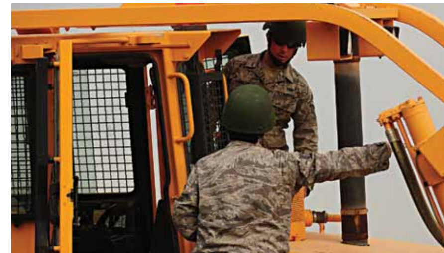
While clearing debris during Operation VIBRANT RESPONSE, TSgt Mark Ordway, site NCOIC, gives direction to SSgt Timothy Yardley. Both Airmen are heavy equipment operators with the 820 RHS, Nellis AFB, Nev. (photo by SSgt Jacob N. Bailey)
