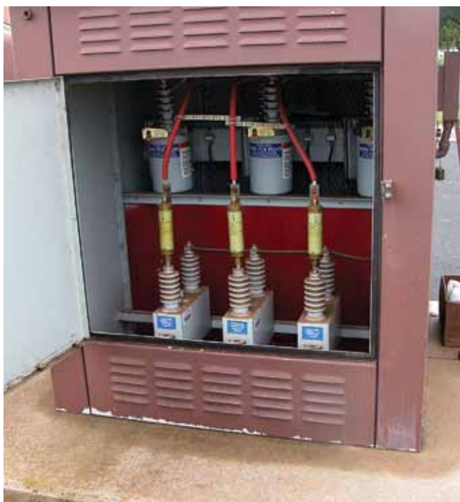
Although they can be installed on underground distribution systems, power factor correction capacitors are often not used with such systems because underground systems have more inherent capacitance than overhead distribution systems. (U.S. Air Force photo)
