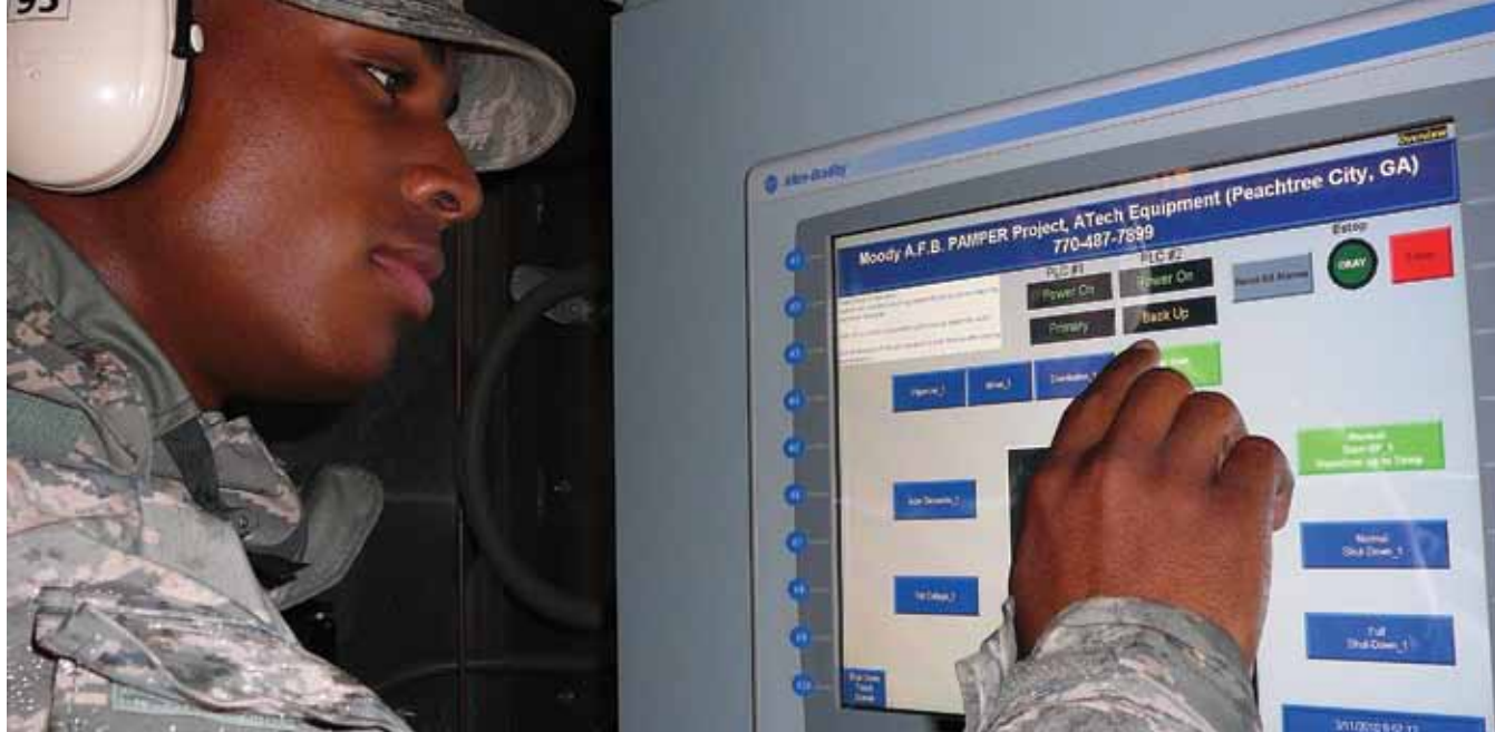
SrA Roderick Gorman, 23 CES, follows an automated checklist to start the plant. (U.S. Air Force photo)
