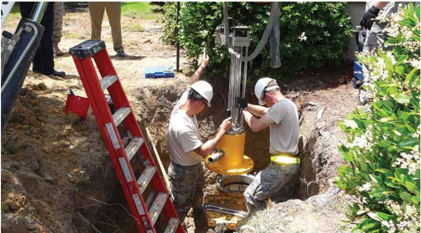
SSgt Jason Reynolds (right) and SrA Patrick Hare of the 23 CES lower the cutting head onto the temporary gate valve to begin cutting pipe for valve insert using the “insert-a-valve” kit. (U.S. Air Force photo)
