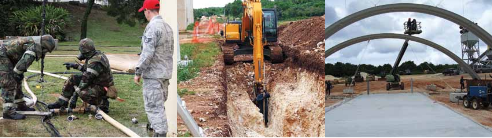
Left: SSgt Kevin Owen, an instructor with Det 1, 554 RHS oversees training at Kadena AB's Silver Flag site. Center and right: A 554 RHS Airman installs utility infrastructure and a combined team of 554th and Guard deployed-for-training CE's construct a K-span at the PACAF Regional Training Center on Andersen's Northwest Field (below).
