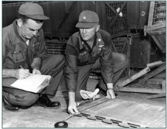
Lt Col Francis E. Torr (right) and MSgt Bruce F. Swafford, members of Prime BEEF Team #1, take measurements on AM-2 in preparation for laying it in aircraft revetments at Tan Son Nhut AB, Vietnam, in August, 1965. (U.S. Air Force photo)
