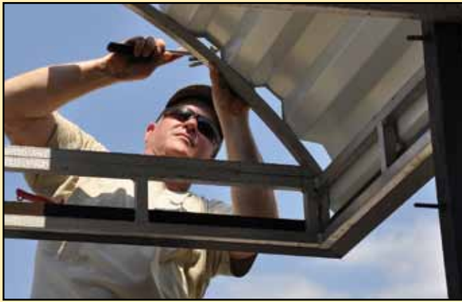
(above top) TSgt Roy Stockinger, a 307 CES (Reserve) structural carpenter, works on an awning on the 307th Bomb Wing Headquarters at Barksdale AFB, La., as part of an on-base renovation project. The 307 CES completed 12 projects at Barksdale worth approximately $250,000 in materials and manhours. (photo by TSgt Jeff Walston)
