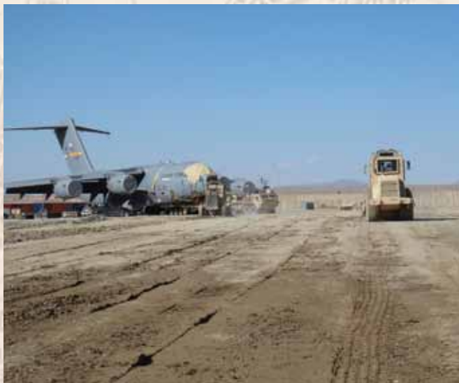
(above) Compaction of soil top course in preparation for AM-2. (photo by TSgt Ursula Rothweiler)
