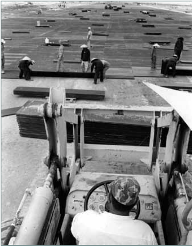
Workers construct a 9000-foot temporary runway of AM-2 at Tuy Hoa AB, Vietnam, in 1966. (U.S. Air Force photo)
