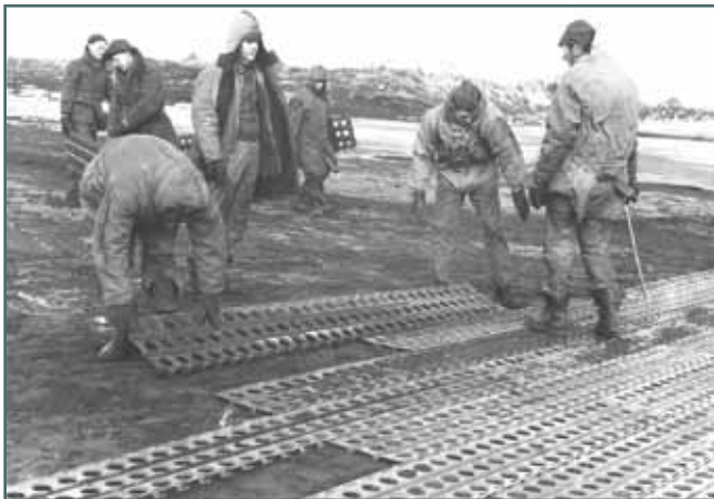
Aviation Engineers in Alaska lay pierced steel plank. The hooks and slots on either side are clearly visible. (U.S. Air Force photo)
