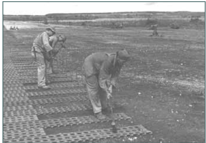
Members of the 804th Engineer Aviation Battalion stake PSP down to the ground during an extension of an airfield to accommodate P-61 "Black Widows" on Saipan in June 1944. The U-shaped clips helped hold the PSP in place during takeoffs and landings. (U.S. Air Force photo)
