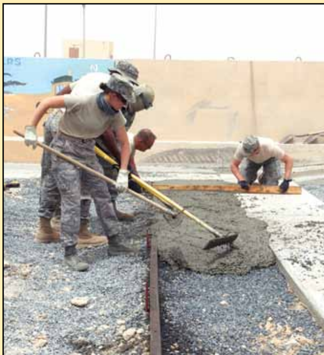
When deployed to the Southwest Asia AOR, civil engineers (here members of the 386 ECES) use the skills honed during home station training projects. (photo by SSgt Alexandra M. Boutte)
