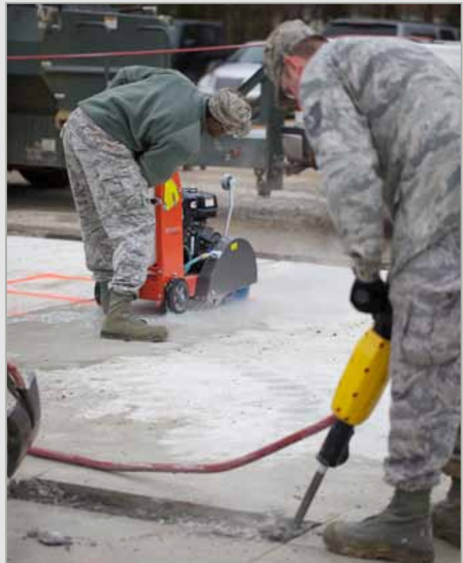
Pavements and Equipment CEs perform a variety of spall and full-depth concrete and asphalt repairs, testing equipment, tools, and materials included in the SuPR Kit. (photo by Mr. Eddie Green)
