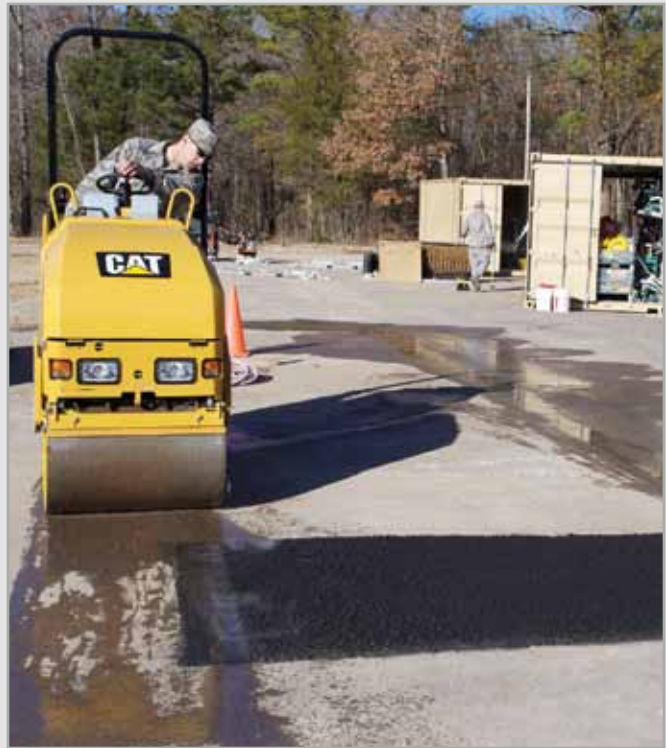
TSgt Jason Collins, 4 CES, Seymour Johnson AFB, N.C., uses the SuPR Kit's vibratory asphalt roller to compact a repaired section of asphalt. (photo by Mr. Eddie Green)
