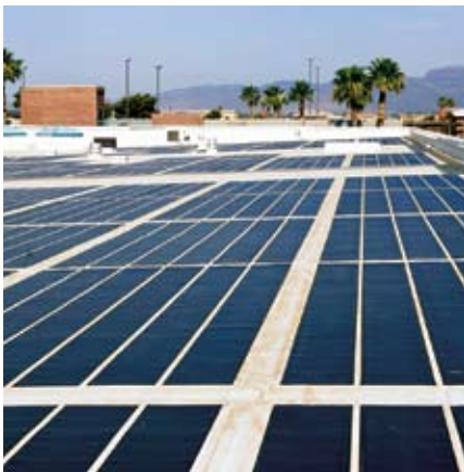
Roof-mounted PV system at Luke AFB (U.S. Air Force photo)
