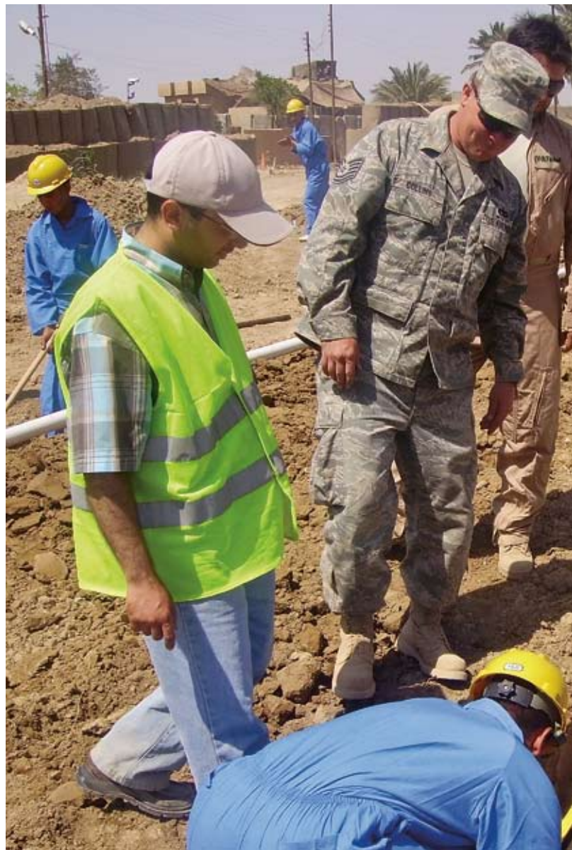
TSgt Chris Collins teaches the Village of Hope plumbing class how to properly install drainage pipe. (U.S. Air Force photo)
