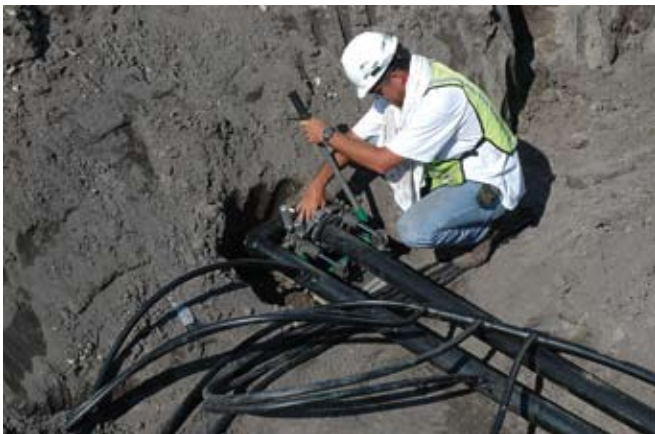
Ground-source heat pump installation at Tyndall AFB (photo by Mr. Guy Ivie)
