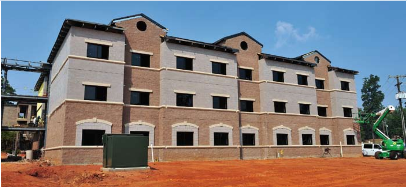
The new dorms at Shaw AFB were built to achieve the U.S. Building Council's LEED Silver certification. (photo by TSgt Josef Cole III)
