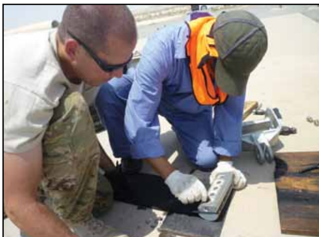
MSgt Jeffrey Stanley of the 557th Expeditionary RED HORSE Squadron works with a member of the host-nation's maintenance crew to attach the aircraft arresting system's new nylon tape during the installation of the overhauled equipment. (photo by SMSgt Stephen Burns)
