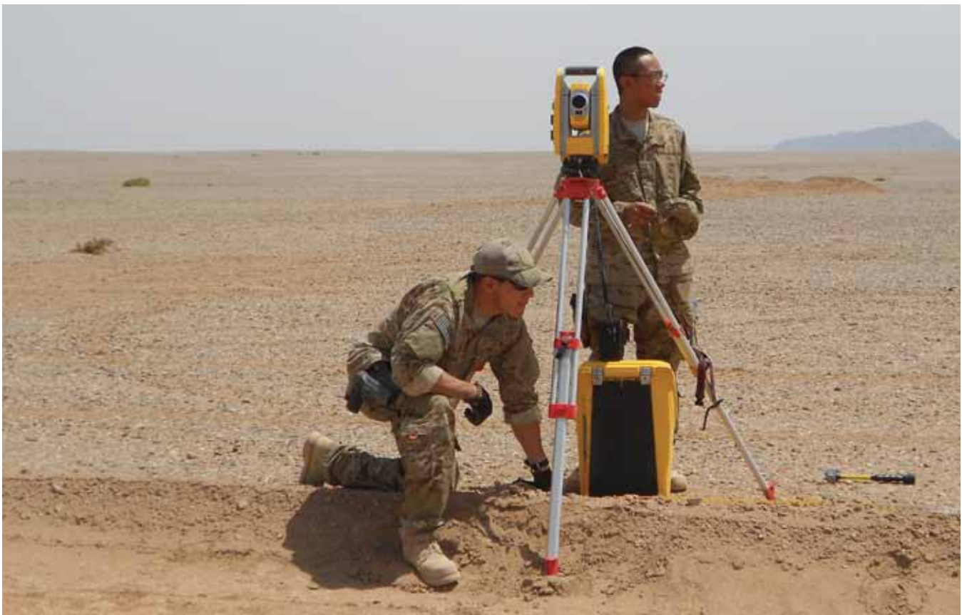
(below) A1C Justin Costa and SrA John Vergara survey the FLS to set grade stakes and determine cut volumes. (U.S. Air Force photo)
