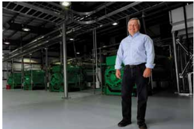
Mr. Tim Berg, 673 CES, stands in front of four electric power generators at JBER's newly constructed LFG power generation facility. (photo by TSgt Brian Ferguson)
