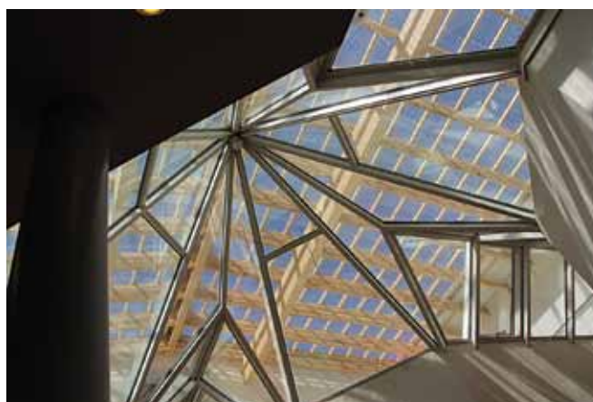
(photos above) The new vented roof on Bldg. 412 protects the area below, including the original skylight, yet still allows daylighting. (graphics and photos courtesy of Mr. Melih Akguenlue, Environmental Chemical Corporation)
