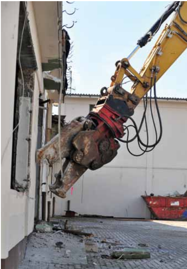
The old base exchange at Ramstein AB, Germany, is torn down using an excavator with a hydraulic shear attachment. (photo by SrA Caitlin O'Neil-McKeown)
