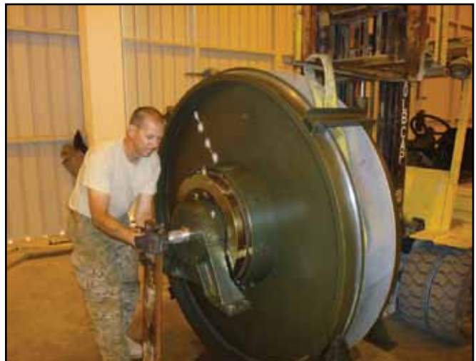
MSgt Jeffrey Stanley of the 557th Expeditionary RED HORSE Squadron prepares a reel assembly to be remounted during the overhaul of one of the airfield's four BAK-12 absorbers. (photo by SMSgt Stephen Burns)
