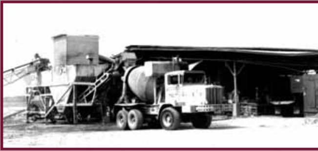
(above) One of two batch plants at Phu Cat which supplied the concrete for a new 60,000 square yard parking ramp. (courtesy photo)
