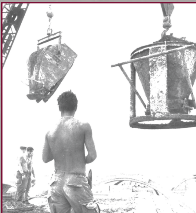
During the Tua Hoa concrete shelter project, craftsmen worked around the clock in sometimes sweltering conditions to finish the project on time. (courtesy photo)
