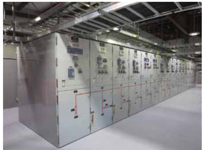
At the power generation plant, switch-gear cabinets transmit power to transformers for final distribution to JB Elmendorf-Richardson (U.S. Air Force photo)
