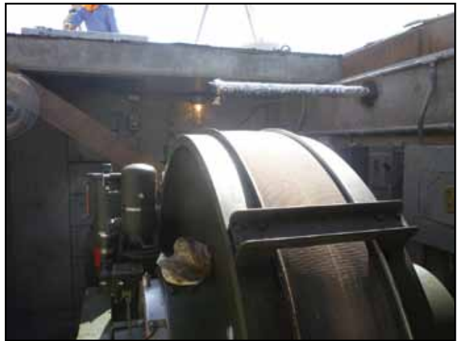
Sections of concrete slab covering the barrier pit are removed in order to access the absorber and lift it from its protective pit for overhaul. (photo by SMSgt Stephen Burns)
