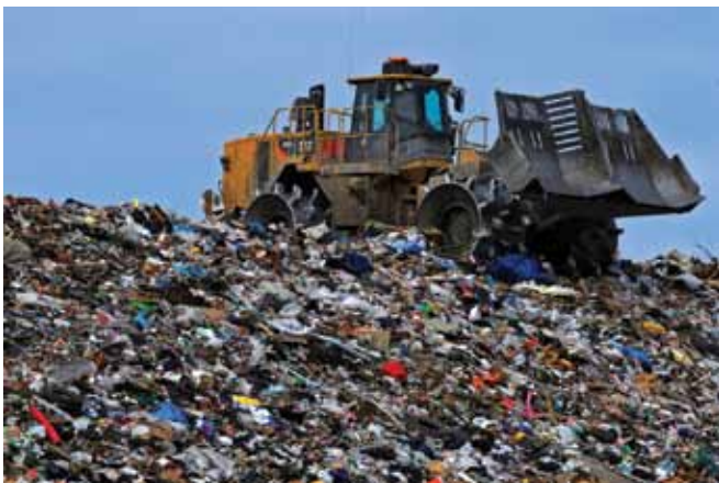
An excavator crushes trash at the Anchorage Landfill in Alaska. Methane gas produced by the landfill is used to generate power for JB Elmendorf-Richardson. (photo by TSgt Brian Ferguson)
