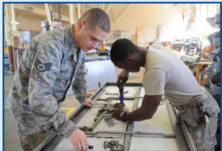
SSgt Anthony Barrow and A1C Tevin Tolver, 2 CES structures, repair a vault door at Barksdale AFB, La. (photo by SrA Kristin High)
