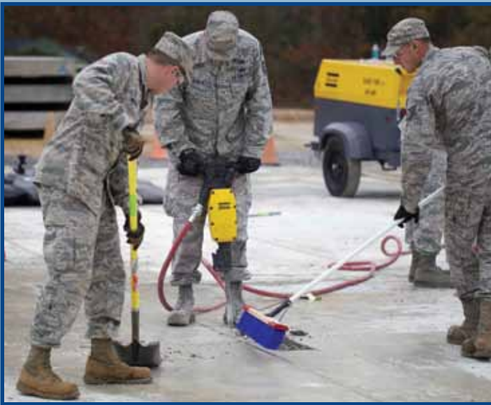
A team of pavements and equipment CEs perform repairs during testing of equipment, tools, and materials included in the new Sustainment Pavement Repair (SuPR) Kit, scheduled to be shipped to the field in 2013. (photo by Mr. Eddie Green)
