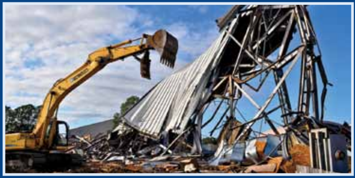
A team uses an excavator to demolish a 1960s-era hangar at Eglin AFB, Fla., to make room for an F-35 fuel cell maintenance hangar, scheduled for completion in 2013. (photo by Maj Karen Roganov)
