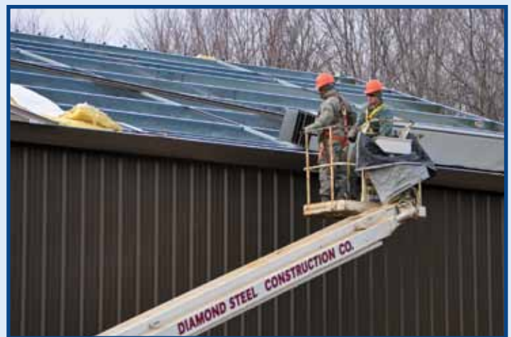
Airmen from the 910 CES, Youngstown ARS, Ohio, construct the roof of a new building for the station's training site on Nov. 14, 2012 (photo by TSgt Brenda Cosola)
