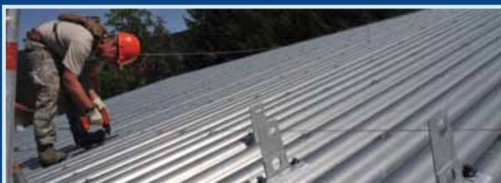
SSgt Robert Parrish, 153 CES, Wyoming Air National Guard, works on a roof snow break installation project as part of annual training. (photo by SSgt Natalie Stanley)
