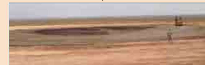
(4.) The Steel Wheel roller compacts the pad. (U.S. Air Force photos by 1st Lt. Matthew Buscemi)
