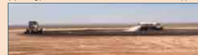
(3.) A grader mixes the SoilTAC, water, Portland cement, and recycled asphalt together. At the same time a water truck sprays the SoilTAC and water onto the center of the pad.
