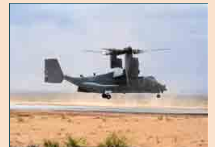
A CV-22 Osprey makes a test landing on the low dust landing pad constructed by the 27th Special Operations Civil Engineer Squadron. (U.S. Air Force photo by Senior Airman Ericka Engblom)
