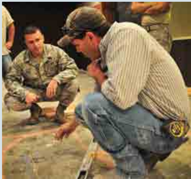
Tech. Sgt. Shaun Lyle, 27th Special Operations Civil Engineer Squadron and another member of the Specialized Maintenance Team work on floor plans for the reconstruction of a lounge at the consolidated club at Cannon Air Force Base, N.M., on Sept. 7, 2012. (U.S. Air Force photo by Airman 1st Class Alexis Pons Abascal)
