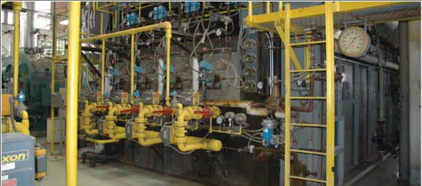
This is one of three central heat plants at Tinker AFB, Okla., scheduled to be decentralized using an Energy Savings Performance Contract. The project could reduce natural gas consumption 40 percent and save up to $7 million. (U.S. Air Force photo)
