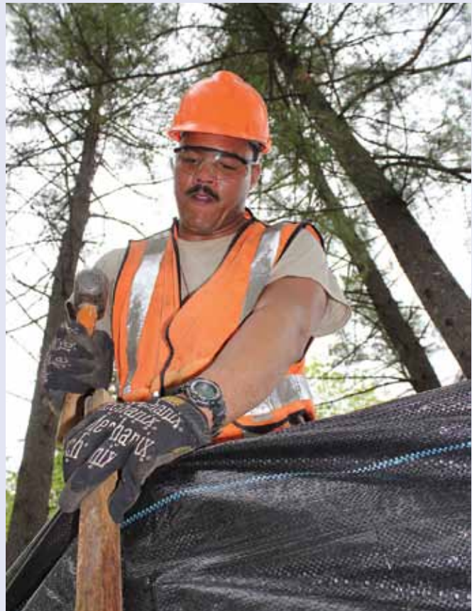
Senior Airman Jason Armstrong pounds in a stake while constructing an erosion control fence at Camp Hinds Boy Scout Camp, Raymond, Maine, May 21, 2014. (U.S. Air National Guard photo/Tech. Sgt. Dan Heaton)
