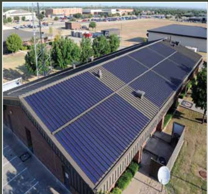
Six sustainable technologies installed atop Goodfellow Air Force Base's security forces building in Texas reduces the utility bill, produces energy and captures rainwater for irrigation. (U.S. Air Force photo/Eddie Green)
