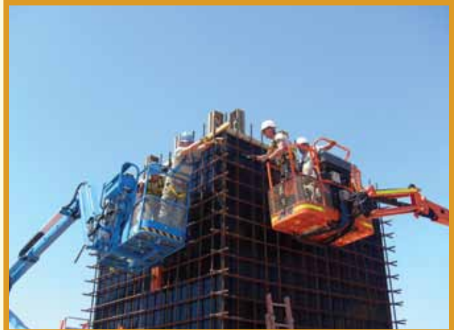
Air National Guard civil engineers deployed to Australia tie rebar on a pedestal for a radar center at Holt Naval Communications Center. (U.S. Air Force photo)
