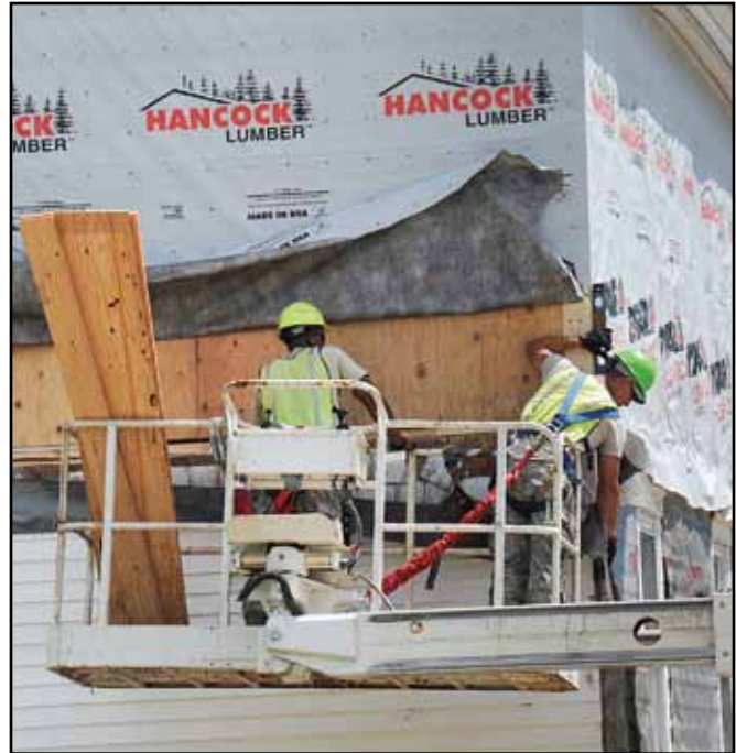
Following OSHA and Air Force guidance keeps safety in the forefront as civil engineers get the job done. (Courtesy Photo)
