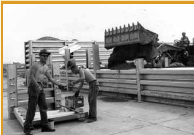
Members of Prime BEEF Team XII construct revetment for F-4C aircraft at Da Nang AB, Vietnam. (U.S. Air Force photo)
