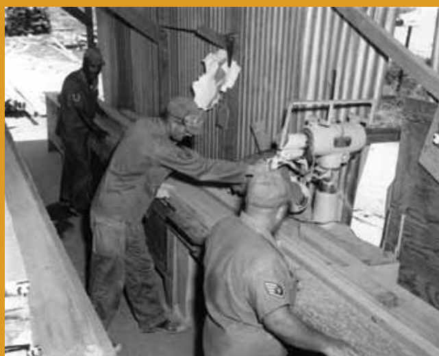
Members of Prime BEEF Team X cut lumber for the construction of barracks at Nha Trang AB, Vietnam. (U.S. Air Force photo)
