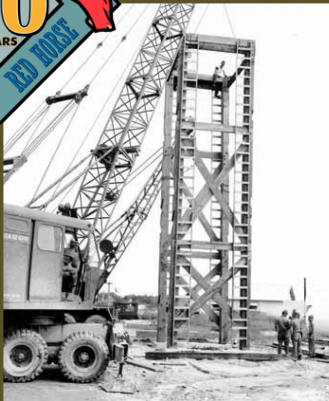
A Prime BEEF team constructs a water tower at Da Nang AB, Vietnam, November 1966.
