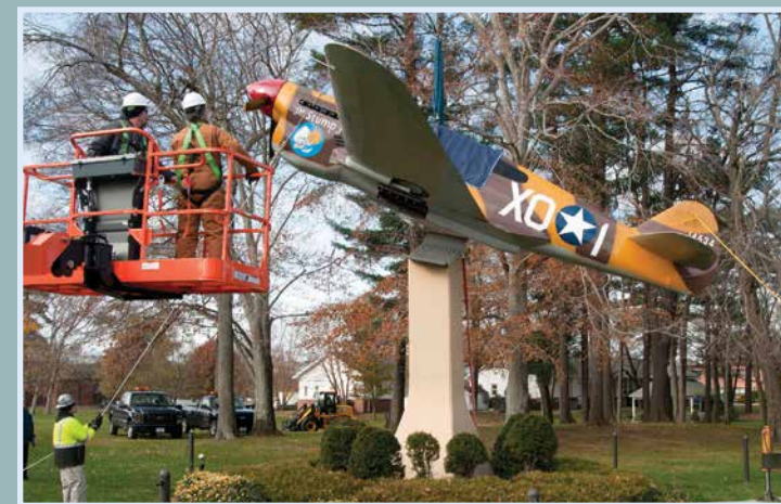
Workers return the P-40 aircraft to its pedestal on the corner of Vandenberg and Marrett streets at Hanscom AFB after the completion of a more than three month-long repair and restoration project by base civil engineers. The model received a thorough sanding and several sheet metal panels were replaced before it was primed and painted. (U.S. Air Force photo by Mark Wyatt/Released)
