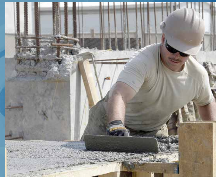
An Expeditionary Prime BEEF Squadron water and fuels systems manager smooths out concrete at a construction site at an undisclosed location in Southwest Asia. (U.S. Air Force photo by Tech. Sgt. Marie Brown/Released)
