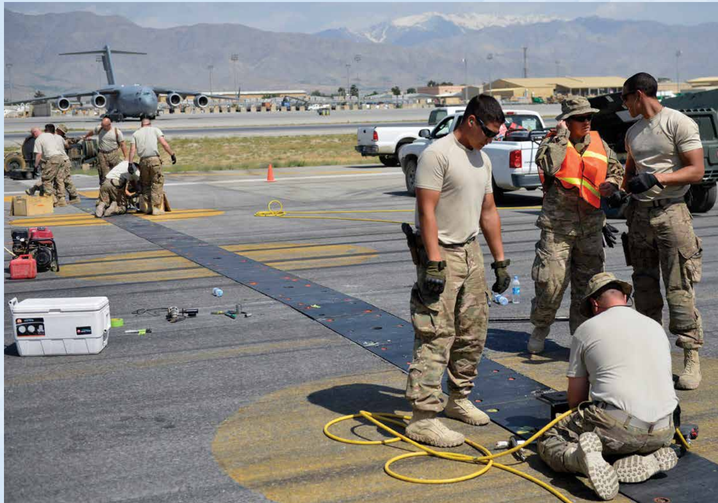
U.S. Air Force Airmen with the 455th Expeditionary Civil Engineer Squadron, grind down bolts on a polly pad on the flightline at Bagram Airfield, Afghanistan. Grinding down the bolts is necessary to prevent aircraft from popping tires when running over the polly pad. (U.S. Air Force photo by Staff Sgt. Evelyn Chavez/Released)
