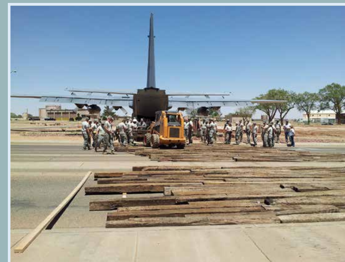
Members of the 27 Special Operations Civil Engineer Squadron, Cannon AFB, NM, build a railroad tie bridge to move an MC-130 static display into place. The MC-130, call-sign "Cherry 01", participated in the legendary Son Tay POW raid and is now on display at Cannon AFB. (U.S. Air Force/courtesy photo)
