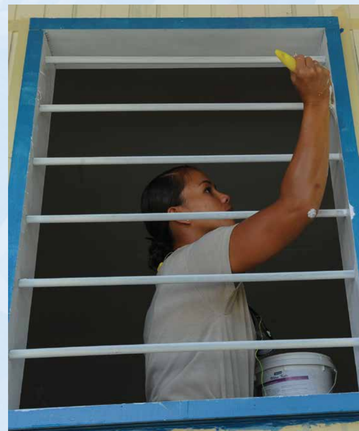
Staff Sgt. Melissa Pascua, 154th Civil Engineer Squadron emergency management journeyman deployed from the Hawaii Air National Guard, paints the window of a newly constructed dormitory as part of Pacific Unity 14-8 in Mount Hagen, Papua New Guinea. PACUNITY helps cultivate common bonds and fosters goodwill between the U.S. and regional nations through multi-lateral humanitarian assistance and civil military operations. (U.S. Air Force photo by Tech. Sgt. Terri Paden/Released)
