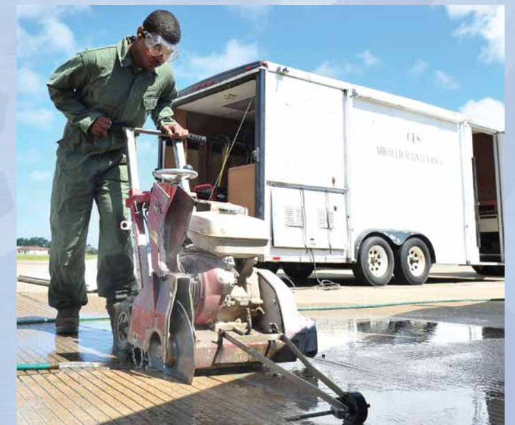
U.S. Air Force Senior Airman DaQuan Price, 633rd Civil Engineer Squadron pavements and equipment craftsman, cuts a section of the runway at Langley Air Force Base, Va., Aug. 27, 2014. The 633rd CES closed the runway to patch damaged areas preventing foreign object debris from damaging aircraft. (U.S. Air Force photo by Senior Airman Connor Estes/Released)
