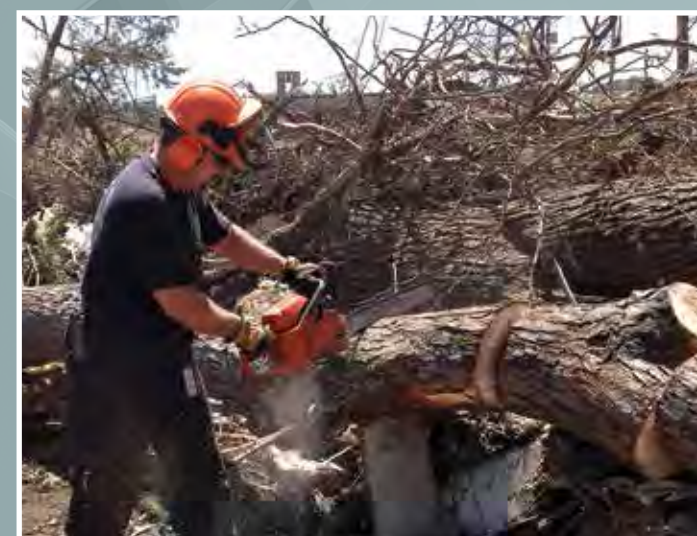
Matt Croteau, a firefighter from the 55th Civil Engineer Squadron at Offutt Air Force Base, Nebraska, cuts debris in Pilger, Nebraska, June 20 with a chain saw. Croteau was part of a group of volunteers from Offutt who helped with the cleanup efforts in Pilger after a tornado destroyed approximately 75 percent of the town June 16. (Courtesy photo)
