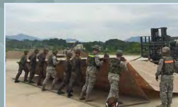
Airmen from the U.S. and Republic of Korea Air Forces work with a large rapid runway repair fiberglass mat during a combined airfield damage repair drill. A foreign-object debris mat is anchored over a repaired hole once a crater is refilled and smoothed. (U.S. Air Force photo/Maj Rueben Choi/released)
