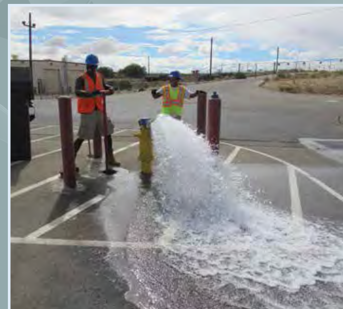
AFMCA engineers provide support for the command's physical plants. Members of the 412th Civil Engineer Group perform a hydrant flow test as part of their preventive maintenance program at Edwards Air Force Base, California. (U.S. Air Force photo/Murray Westley/released)
