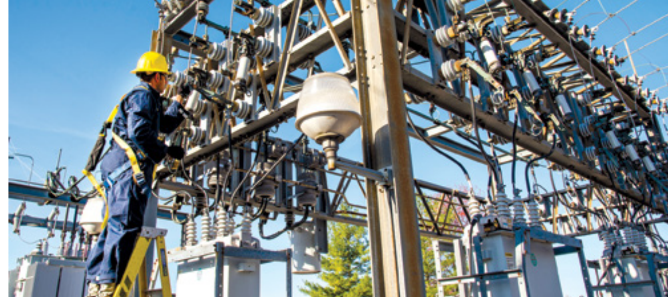
Staff Sgt. Manoj Williams, 375th Civil Engineer Squadron electrical systems craftsman, greases framework knife blades and tightens loose conductor connections in April 2016, at Scott Air Force Base, Illinois. The base required a scheduled power outage to repair critical high-voltage electrical components. A recent grid security exercise tested North America's preparedness plans. (U.S. Air Force photo by Airman Daniel Garcia)
