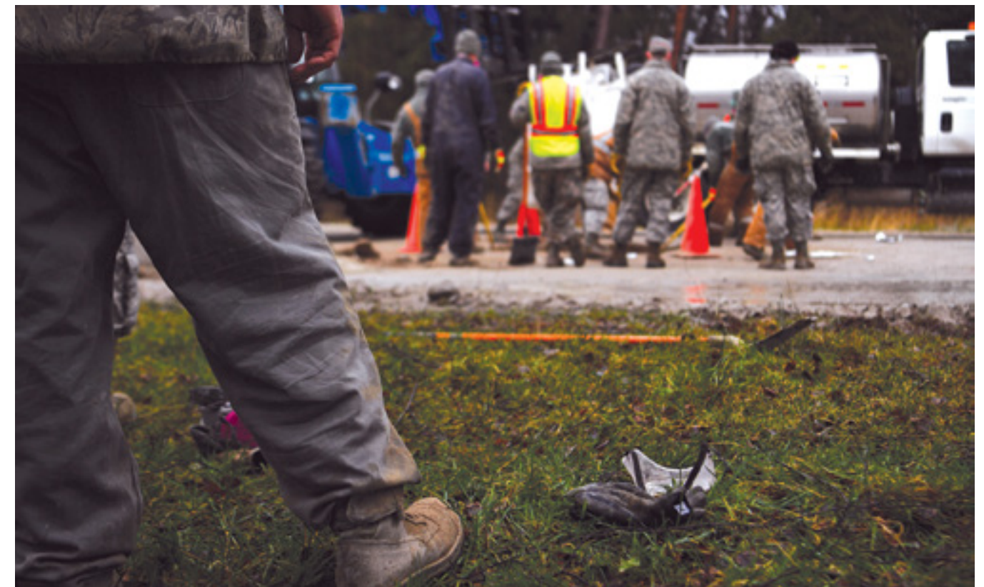
ABOVE: A U.S. Airman watches as his counterparts fill a hole in the runway during a RADR training exercise on Ramstein Air Base, Germany, Jan. 25, 2018.
