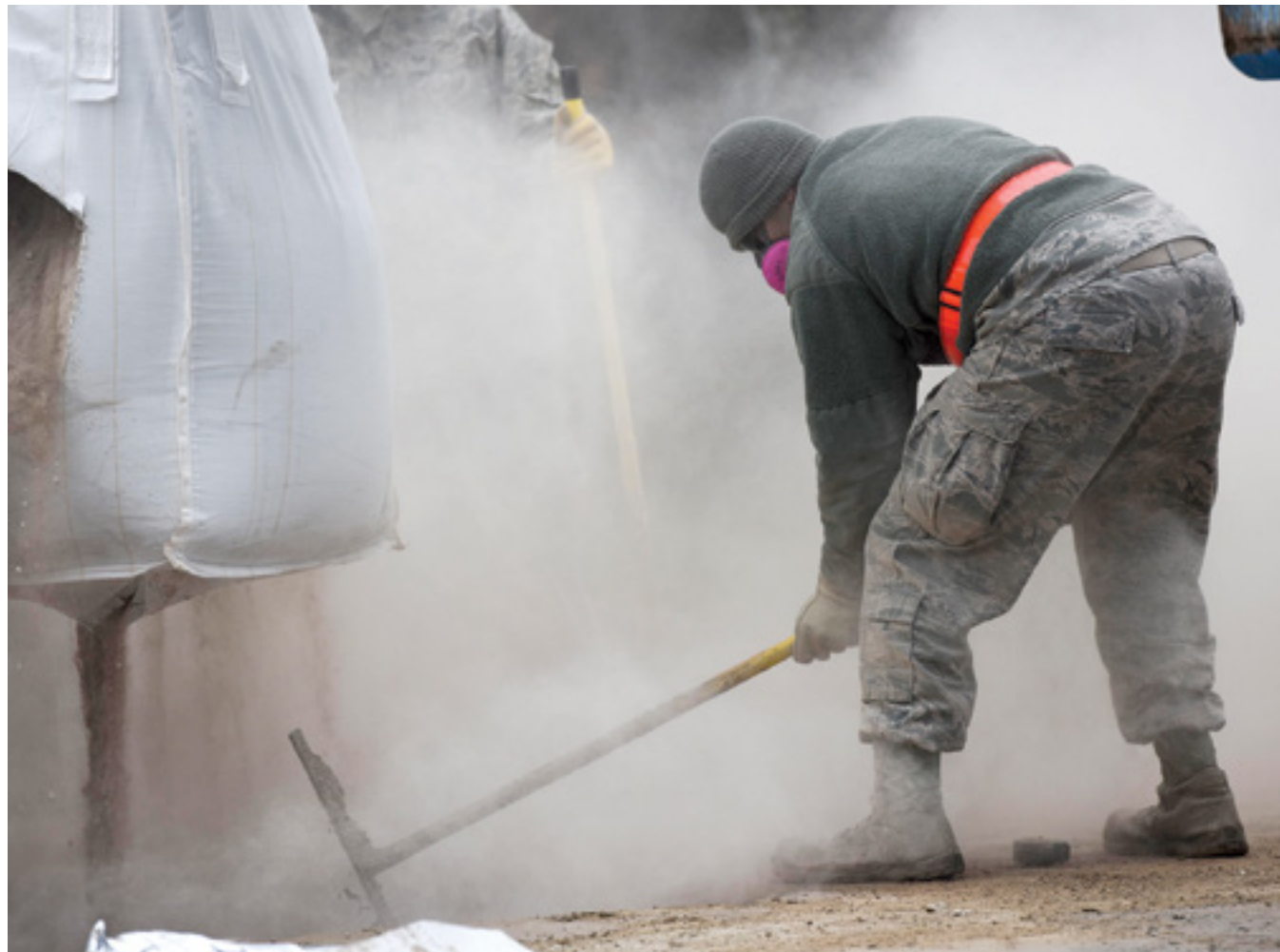
U.S. Air Force Staff Sgt. Antonio O'Campo, 773rd CES electrical systems journeyman, mixes flowable fill concrete for a RADR training exercise on Ramstein Air Base, Germany, Jan. 25, 2018. O'Campo was part of the first class to be trained in the updated RADR course. (U.S. Air Force photo by Senior Airman Devin M. Rumbaugh)
