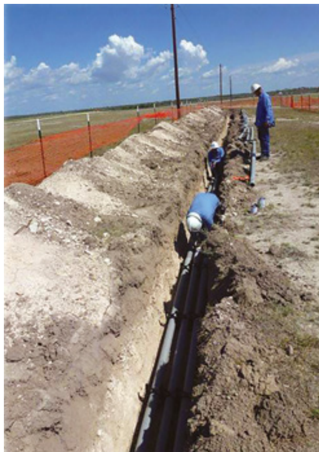
Crewmen from the Rio Grande Electrical Cooperative place new electrical cables underground at the south end of the flight lines as part of the overhead-to-underground electrical distribution conversion project at Laughlin Air Force Base, Texas, in November 2012. Underground systems can be beneficial near airfields. (Courtesy photo)
