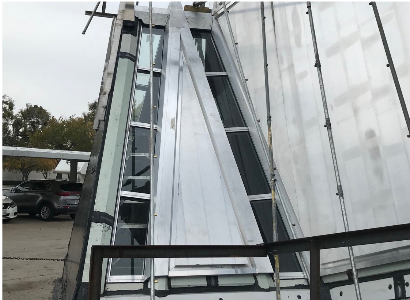
A mock-up of the middle tetrahedron joint area of design of the U.S. Air Force Academy Cadet Chapel in Colorado Springs, Colorado. (U.S. Air Force photo by Megan P. Robare)
