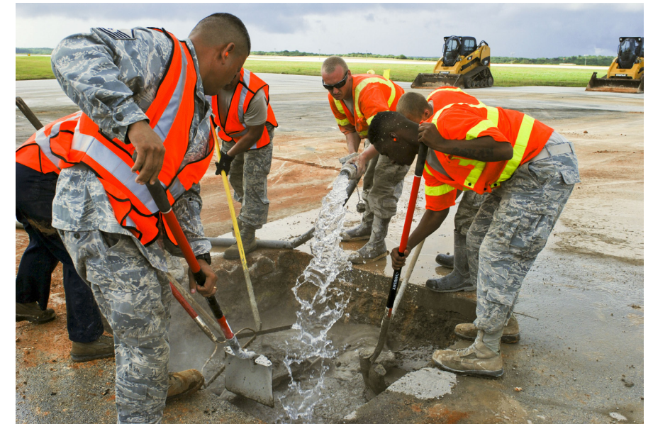
Airmen from the 36th Civil Engineer Squadron mix water and a low-strength concrete together in the area where simulated damage was created during an airfield damage repair training exercise on the Andersen Air Force Base, Guam, flightline Jan. 23, 2014. The 36th Civil Engineer Squadron Airmen were the first in the Air Force to receive training on a new airfield damage repair capability. (U.S. Air Force photo by Airman 1st Class Emily A. Bradley)
