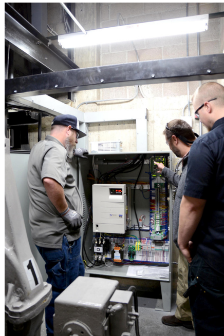
James "JT" Trantham, contracting officer representative, center, explaining to stakeholders the functionality of the new control system with the help of the onsite elevator contractors Robert Hanson, left, and Kyle Munson. (U.S. Air Force photo by Master Sgt. Jasmine Reif)
