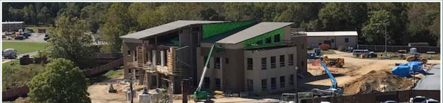
Malcom Grow Medical Clinic and Surgery Center – Phase 2 Construction (U.S. Air Force photo)
