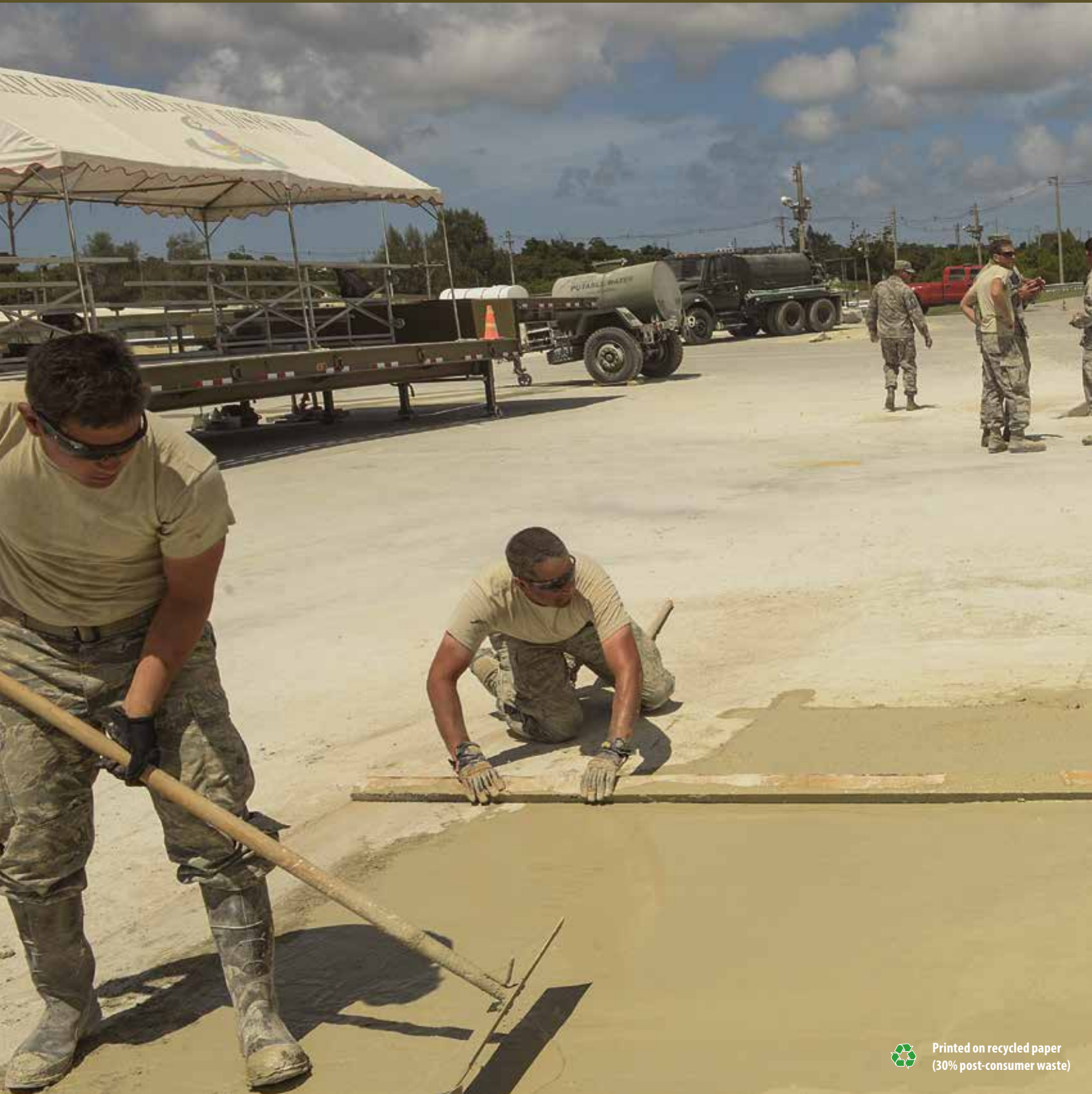
U.S. Airmen assigned to the Kadena, Yokota and Misawa civil engineer squadrons practice concrete screeding skills using the materials, equipment and methods to repair craters during airfield damage repair training exercise at Kadena Air Base, Japan, Sept, 15, 2016. This process can be done quickly in combat situations so airfield operations can resume. (U.S. Air Force photo/Senior Airman Stephen G. Eigel)
