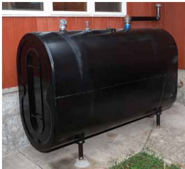
Example of outdoor above-grade fuel storage tank.
