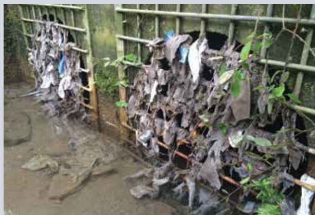
Debris from a sewage overflow is seen attached to a grate covering the outflow pipe.
