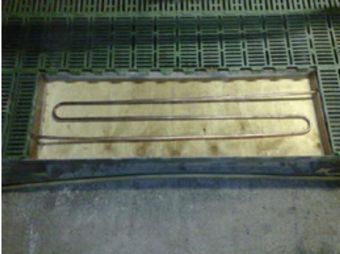
Figure 9. Typical copper pipe 'S' shaped section prior to pouring one of the concrete heating pads in the piggery farrowing sheds.
