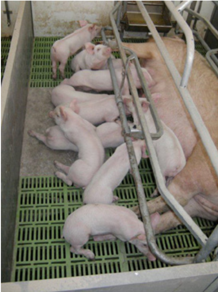
Figure 10. Farrowing pen at the Grantham piggery showing one of the concrete pads heated by circulating hot water through copper pipes cast into the pad.
