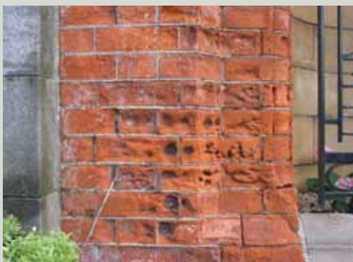
Weathering of brickwork can in some cases be severe. In this case, the decay may have been exacerbated by the mortar being too strong
