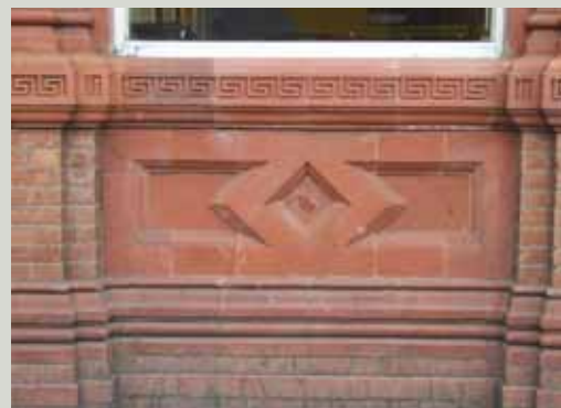
This terracotta panel has been carefully repaired following the removal of an automatic teller machine which had been inserted beneath the window
