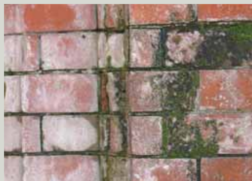
Soluble salts visible on the surface of this brickwork have been caused by rising damp in the wall. The moss growth present is another symptom of the excessive dampness of the bricks the cause of which needs to be diagnosed and treated
