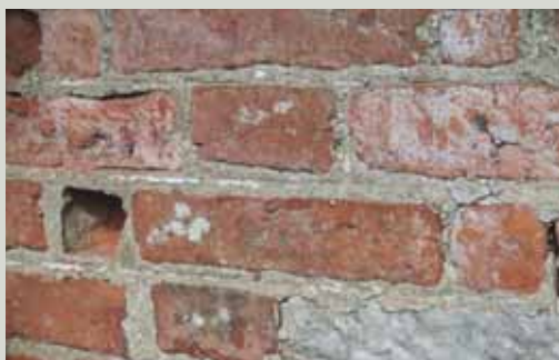
Colour washed bricks with traces of pencilling to the joints at the Hell Fire Club, Desmond's Castle, Askeaton, Co. Limerick
