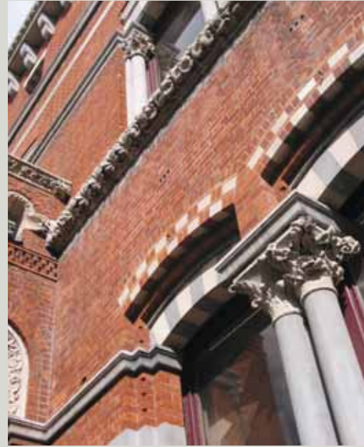
The decorative brick and stone façade of the former Kildare Street Club, Dublin designed by Deane and Woodward and built in 1859-61
