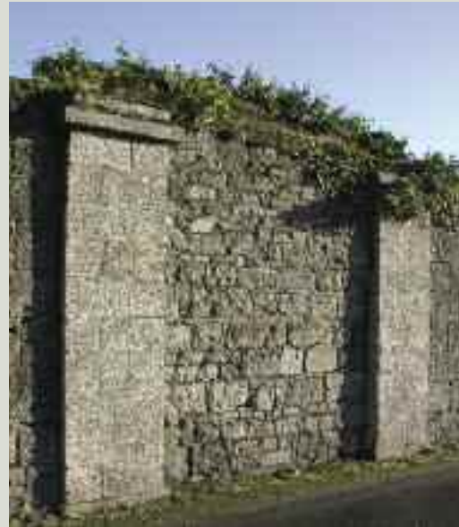
This image highlights the contrast between the finely worked stonework of the ashlar piers, with narrow joints between the stones, and the coursed rubble walling that was used to block up the former gateway between the piers
