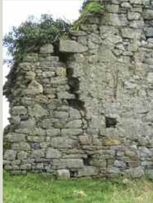
Tapering cracks can result from subsidence. As the crack widens the smaller stones fall out or drop inside the wall creating a wedge effect and increasing the damage
