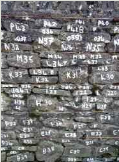
Masonry wall with stones numbered to allow for accurate rebuilding. The strings are stretched across the length of the wall to mark the wall at vertical intervals to ensure joints are kept at original thickness when rebuilding
