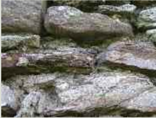
Decayed/weathered lime mortar
