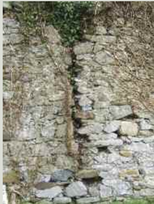
Vertical cracks can be more common in walls where few long facing stones were used. Longer stones create a stronger bond than smaller stones
