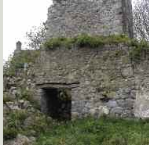
The condition of the surrounding masonry is important in the survival of timber lintels. If the wall top or pointing is poor, water will lodge on top of the timber lintel and cause decay
