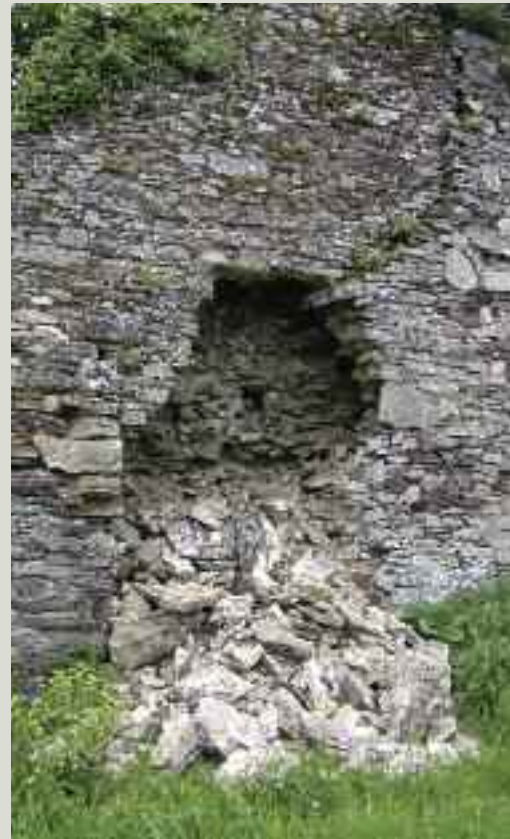
A partial collapse of the town wall of Youghal, County Cork. Recently-collapsed structures should not be approached until after a structural engineer has deemed it safe to do so
