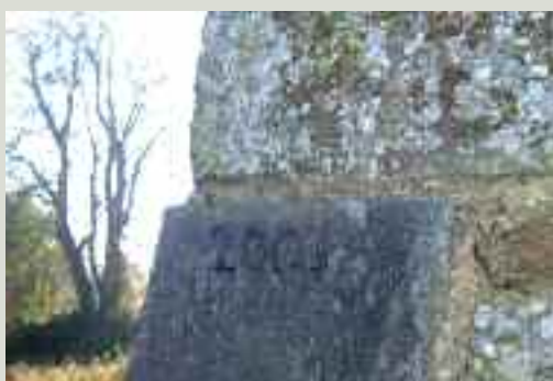
A date has been etched into the stone to distinguish the new stone from the original
