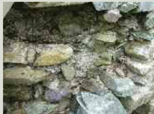
Wall with its outer face lost exposing the construction of the wall core
