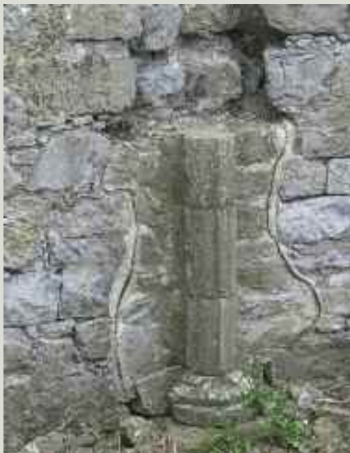
A method of distinguishing between old and new masonry in repair work was used by the Office of Public Works in the mid-twentieth century and can still be seen on many national monuments today. The technique involved separating the new from the original by the insertion of a strip of felt. This technique is no longer used today
