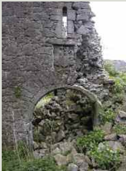
Partial collapse of this church tower occurred suddenly, taking down a portion of the nave wall
