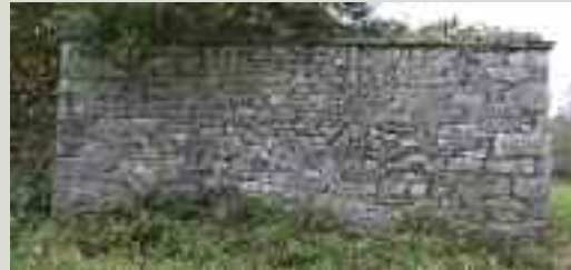
Uncoursed random rubble. Note the large quoin stones at the corners which give strength to the structure
