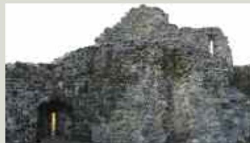
A repair to a town wall using new stone where the wall had been damaged or robbed. In this case, the new stone was sourced from a quarry 8 km away and, in the course of time, will weather in
