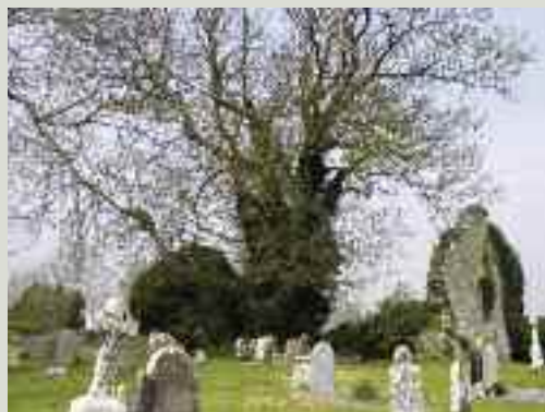
Mature trees adjacent to a ruin present a challenge. While they may add greatly to the beauty, character and natural heritage of a site, they can cause damage by undermining the foundations with their roots, or by falling branches
