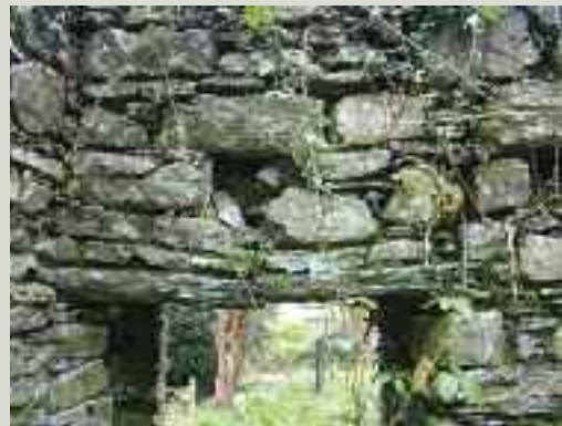
Lintel failure in this case was probably the result of the loss of mortar and stone from the wall above the lintel which damaged the natural self-arching tendency of the masonry placing excessive loading onto the lintel
