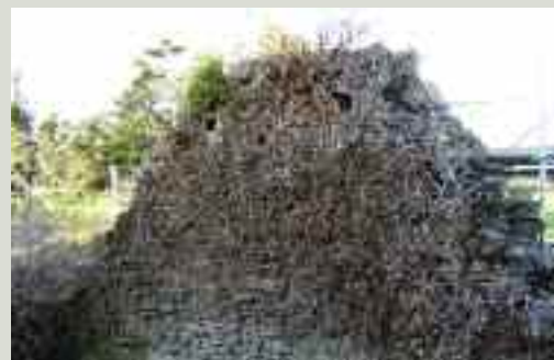
The top layer of vegetation has been sprayed and killed off pending its removal. The treatment allows for assessment and recording of the masonry
