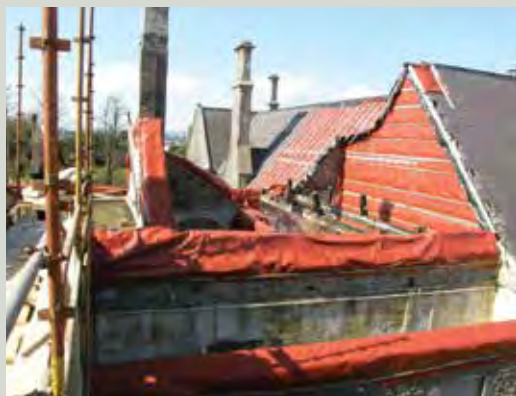
A fire in a nineteenth-century school building destroyed much of the roof. The exposed wall tops, gables and junctions with the surviving roof were temporarily protected against further water damage by fixing a membrane
