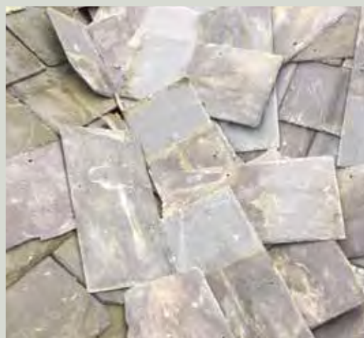
Detail of slates stripped from a roof and piled up at the bottom of the valley gutter
