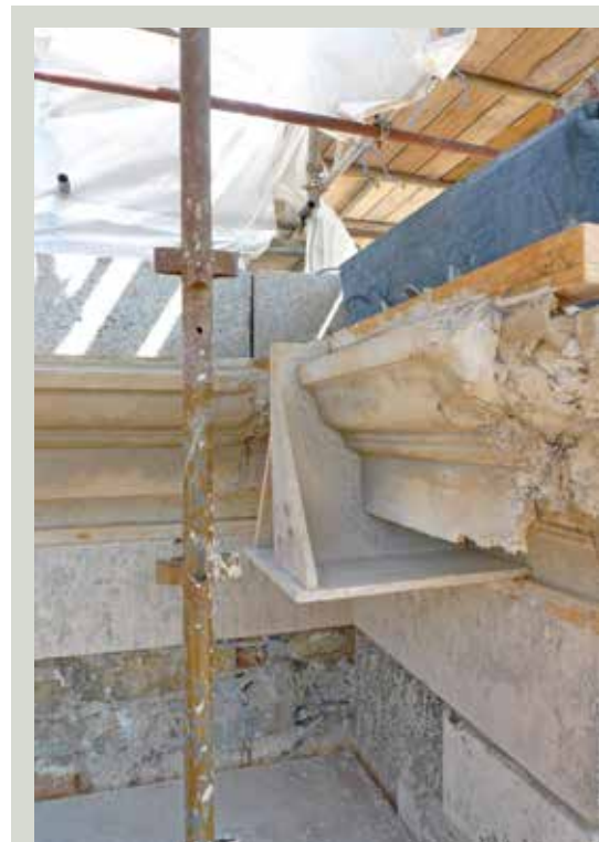
Carrying out repairs to a historic building requires an experienced contractor capable of undertaking specialist work such as running this plaster cornice in situ (Image courtesy of ARC Consultants)
