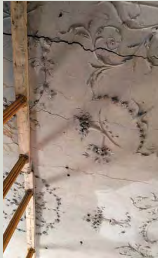
Most of this significant rococo ceiling was saved in the immediate aftermath of a fire by drilling holes to release fire-fighting water trapped above and by providing propping
