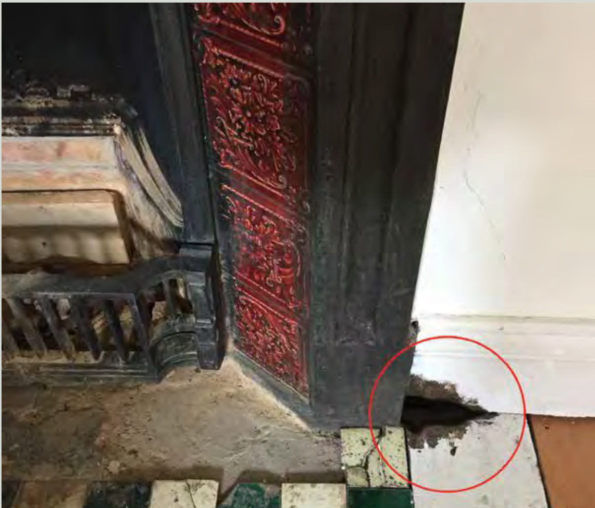
A traditional cast iron fireplace where glowing soot fell behind the fireback and began to burn the floor and skirting (circled) adjacent to the fire surround
