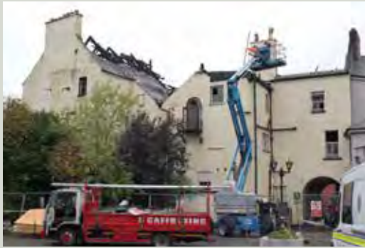
Potentially unstable features such as chimney stacks being made safe following a fire to prevent further collapse and damage
