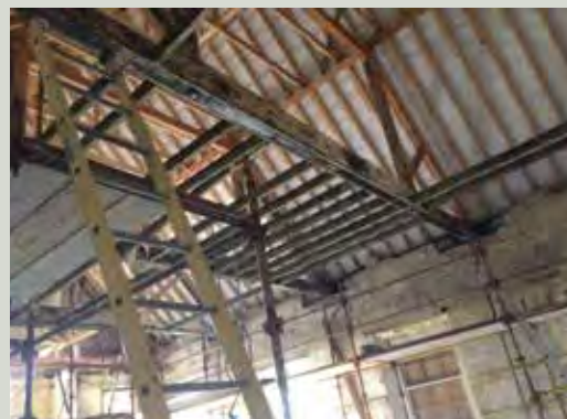
These timber trusses were left exposed to the weather for five years following a serious fire. On examination, they were found to be generally sound and were retained in the re-roofing works supplemented by the addition of new timber members. Detached wall and ceiling plaster can be re-secured; damaged structural timbers can be repaired in-situ
