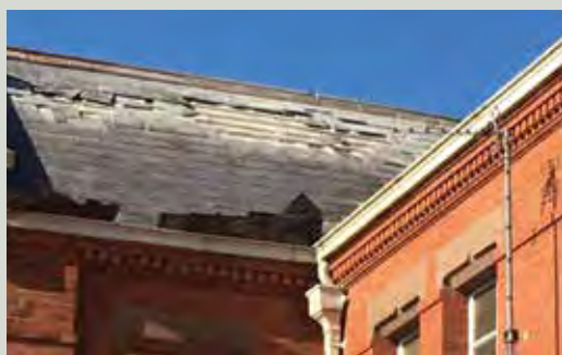
These images are examples of damage during a severe storm in 2017. When a breach is made, the wind gets under the roof covering and lifts it off. Had the storm lasted for longer, entire roofs might have been stripped
