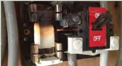
A burnt-out switch on left indicates overloading
