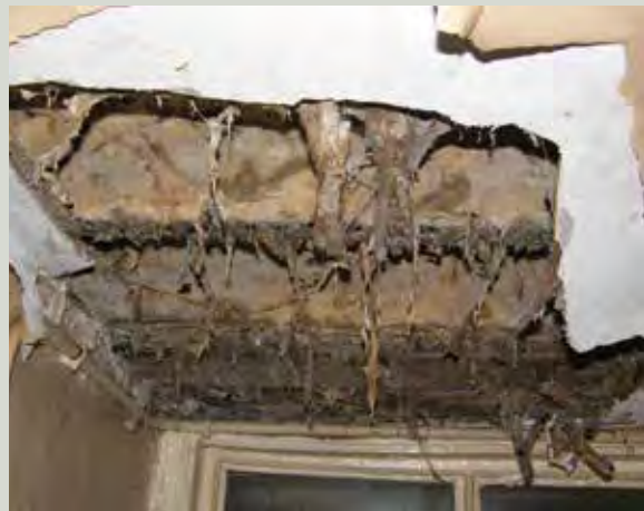
The underside of a timber floor with a severe outbreak of dry rot
