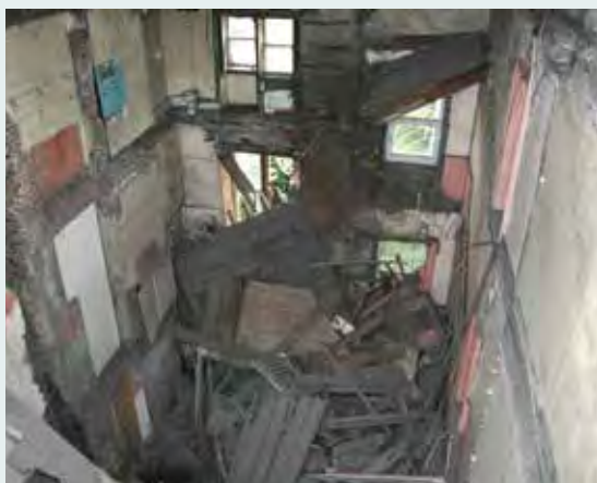
Catastrophic collapse of historically important but vacant building in which the entire internal structure fell in because a spine wall collapsed at a lower level (Images courtesy of Cork City Council)
