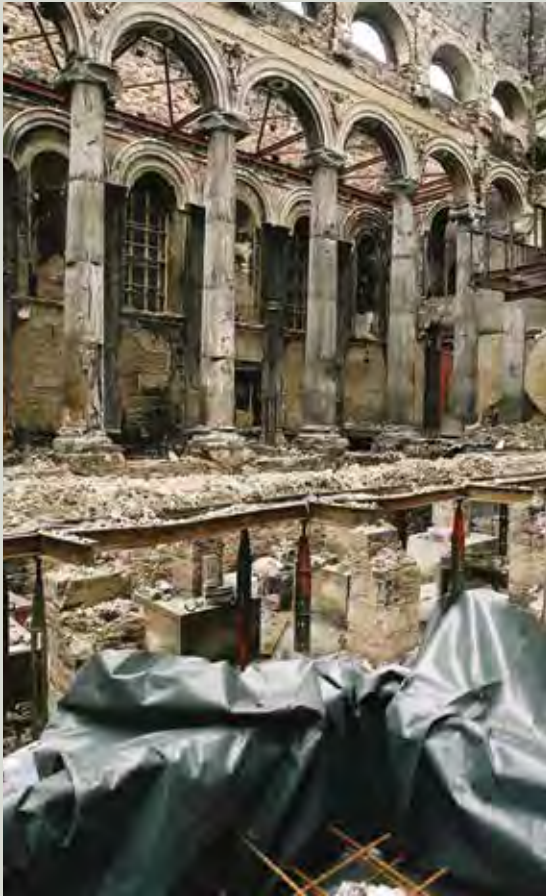
Urgent temporary works carried out included installing props to the floor structure and bracing between walls at high level as well as covering artefacts with plastic sheeting
