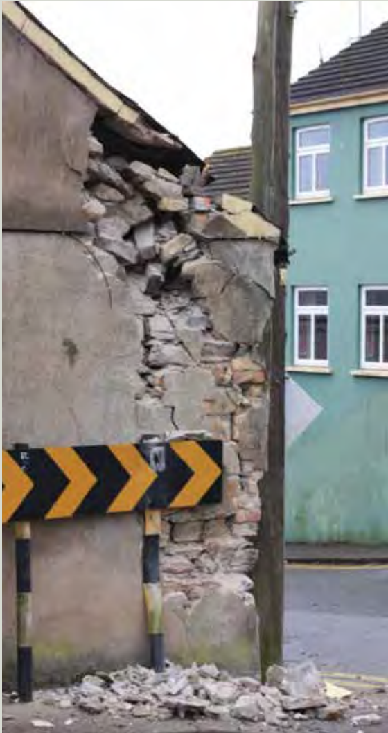
The damage to the gable after the vehicle was removed. The wall was rebuilt using the salvaged material from the mid-point of the gable to the windows on the front wall. A simple bollard would offer protection here. In previous centuries, jostle stones were used to prevent impact from horse-drawn vehicles
