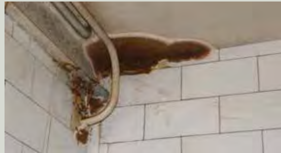
A slow leak from water pipes has caused this outbreak of dry rot
