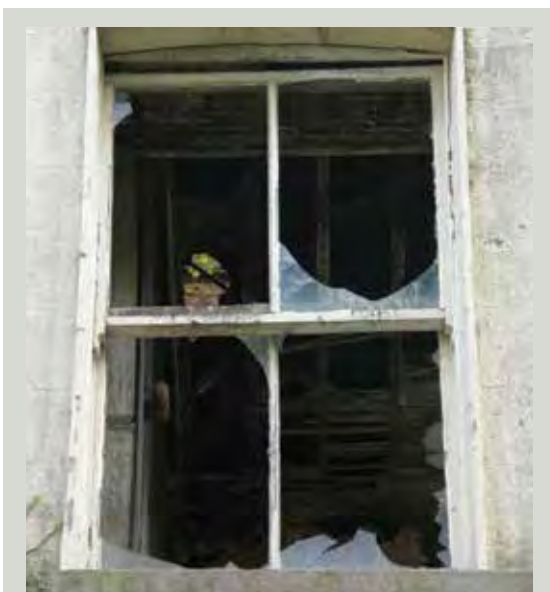
Broken window glass leaves a building interior exposed to water ingress and will increase the risk of rot at floor level. If left unrepaired, it may attract further vandalism
