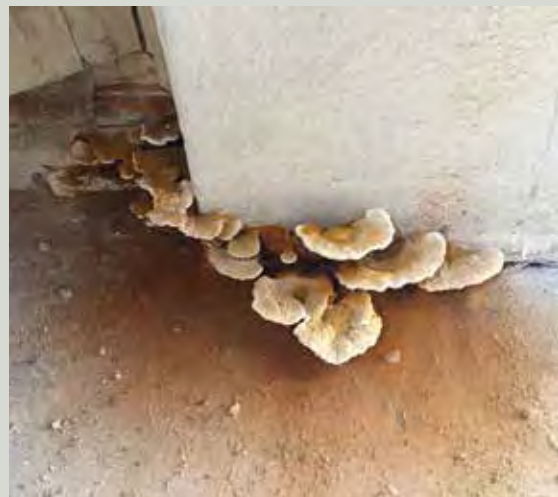
An outbreak of dry rot in the floor became obvious a few years after the building had been reroofed following a period when it was open to the elements after a fire
