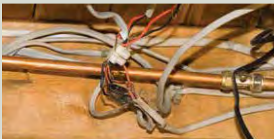
Against all regulations and good practice, this electrical wiring is jointed with an inadequate and unsuitable connector block. Insulating tape has been used to cover exposed cable. Note the new copper pipe indicating the work was done here relatively recently. Dangerous electrical wiring beside a copper water pipe is a potentially deadly mix
