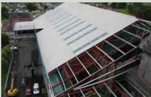
An industrial-type temporary roof was fitted to St Mel's Cathedral to facilitate the programme of conservation works and also to prevent further damage (Images courtesy of FKP Architects)
