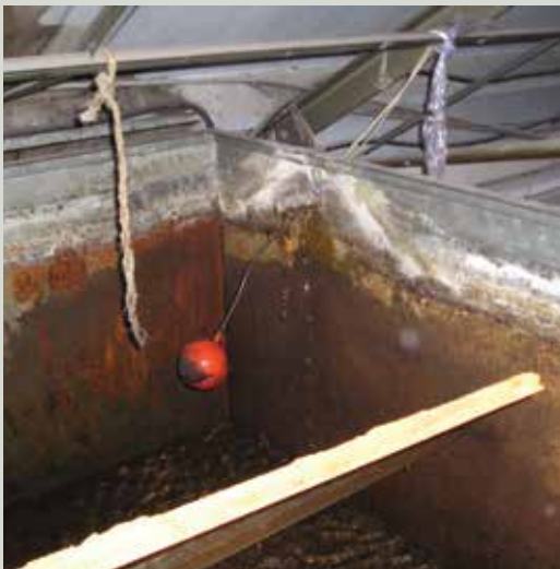
A galvanised steel tank which has been emptied and is showing signs of corrosion. Steel will corrode at different rates depending on the pH of the water. Such a tank can fail suddenly and cause serious water damage as it will continue to take in and leak water until the incoming mains supply is turned off
