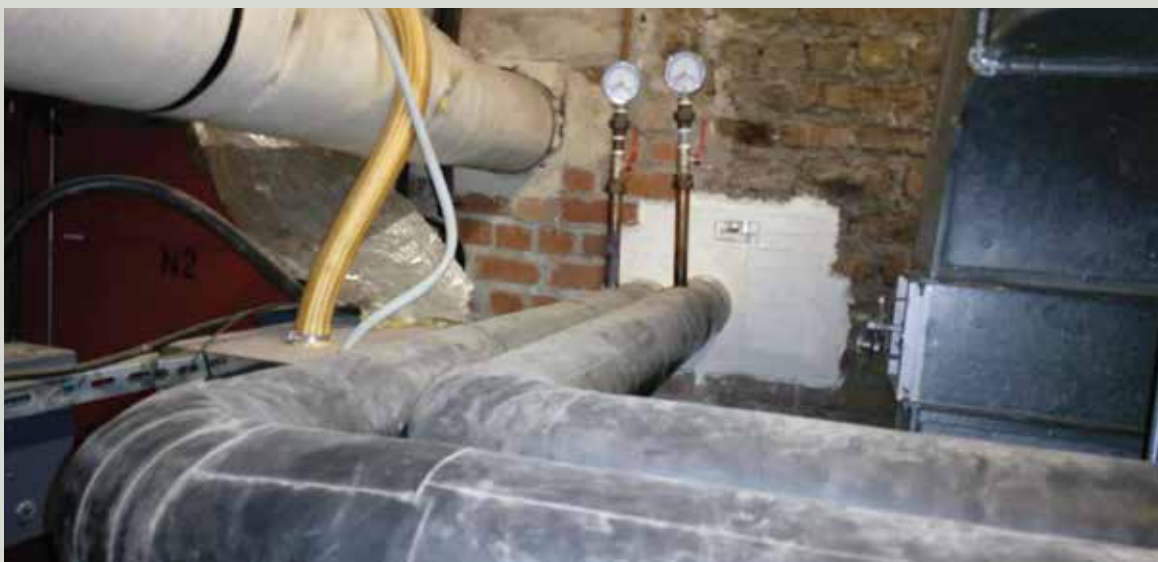
Fire-stopping (white patch) where pipes run through compartment wall
