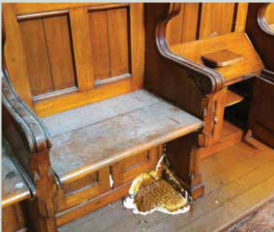
Dry rot fruiting body with its source in the floor under choir stalls in a nineteenth church
