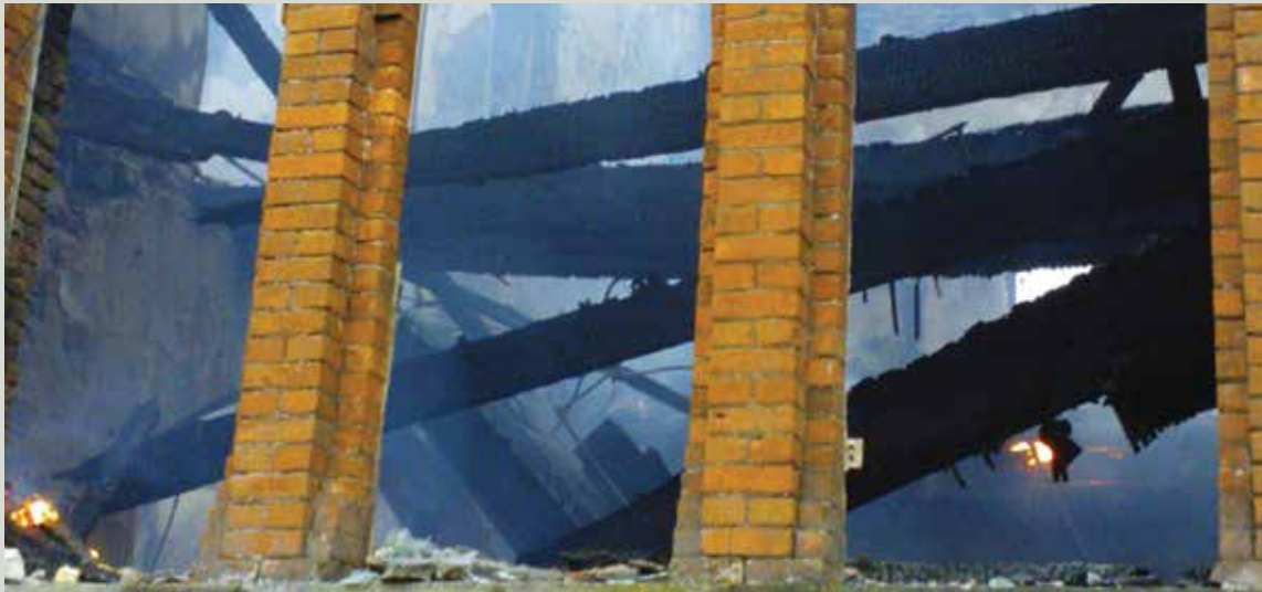
A close-up view of the collapsed floors in the central bay of the same building
