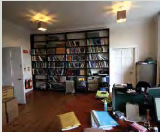
An eighteenth-century Georgian house now in office use. The partition is carried by the floor joists, its weight is increased significantly by the bookcase. Note the distortion in the door and frame to the right caused by the overloading
