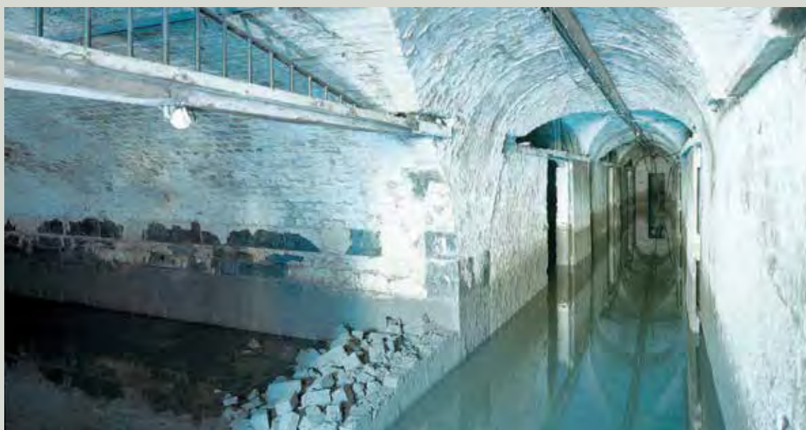
Basements can be particularly prone to flooding (Image courtesy of ARC Consultants)
