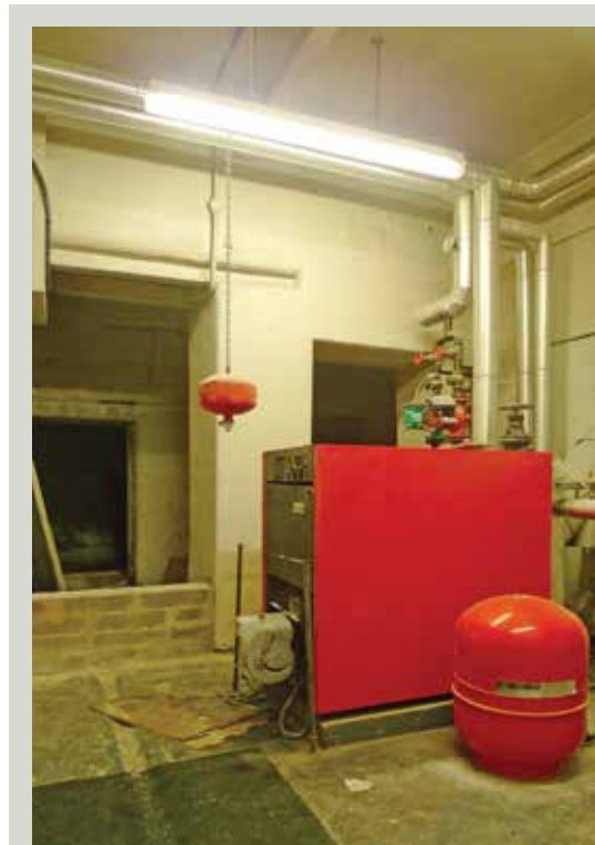
This boiler room is fitted with a hanging dry powder fire extinguisher which will activate automatically in the event of a fire reducing the risk of fire spread (Image courtesy of ARC consultants)
