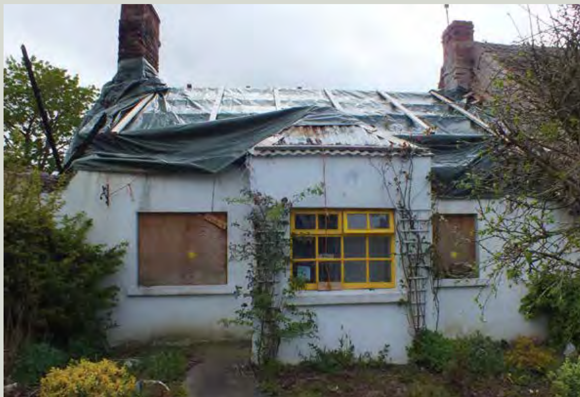
A simple temporary roof of plastic sheeting on the surviving portion of a thatched cottage. Note that the chimney in the foreground had been rebuilt before the fire (Image courtesy of Limerick County Council)
