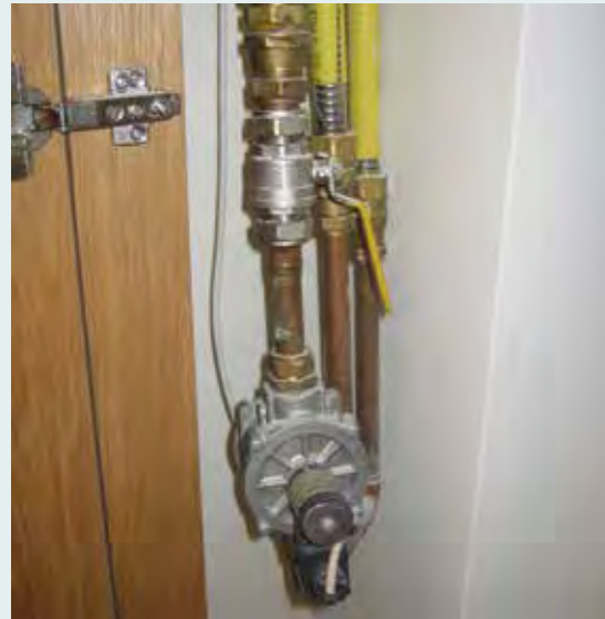
A manual gas valve with yellow handle and an automatic slam-shut valve (bottom) with power cable activated by the alarm system
