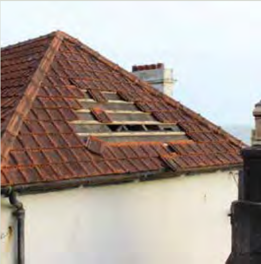
In older tiled roofs, the tiles are simply laid in place. The lugs on the back of the tile hang over the battens without any fixings. Such roofs can suffer more extensive damage in high winds than slated roofs
