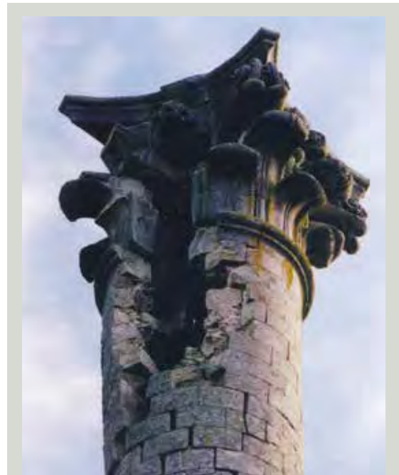
The Browne-Clayton Monument, County Wexford where the force of a lightning strike dislodged masonry at the top (Image courtesy of Rainey's, Swords)
