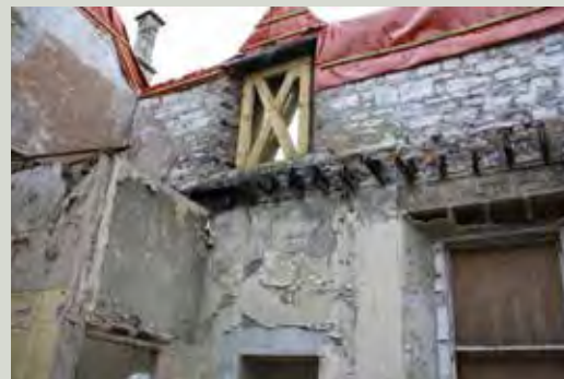
Following a fire, vulnerable openings were braced against movement to avoid further loss of fabric
