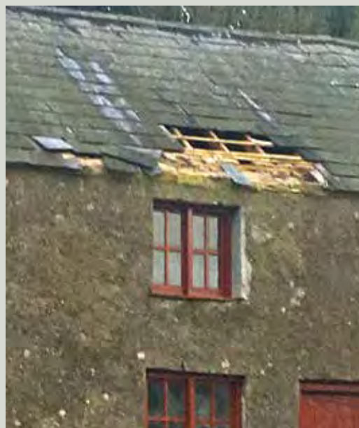
A nineteenth-century farmyard building with no gutters. The wind got under the projecting eaves and blew off the slates
