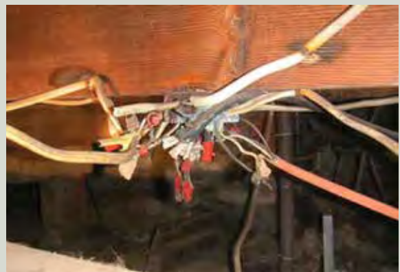
An extremely dangerous assembly of old wiring. Note the scorch marks on timber joists
