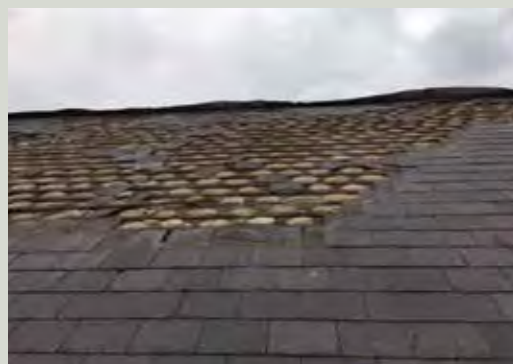
The upper part of this roof has been almost fully stripped and the lead ridge has been blown back
