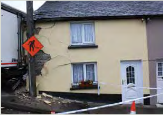
The corner of a small eighteenth-century building immediately after being struck by a truck
