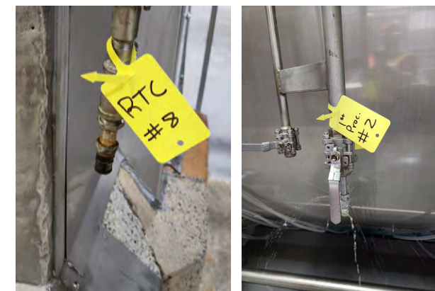
Butterball's Energy Tag Program identifies potential sources of air, steam and water leaks across our six processing facilities that are “tagged” by our maintenance teams.
