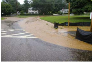
R. Schnabel, Chesapeake Bay Foundation Sediment laden runoff pouring off the construction site
