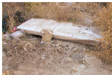
US Environmental Protection Agency Storm drain filled with trash and debris
