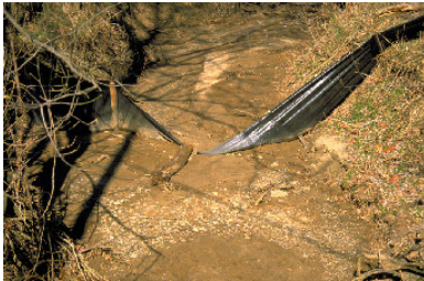
US Environmental Protection Agency Failing silt fence (Runoff pools at a low point and can overwhelm a silt fence.)
