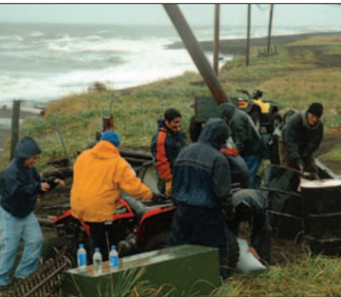
Residents right a utility pole during a storm.
