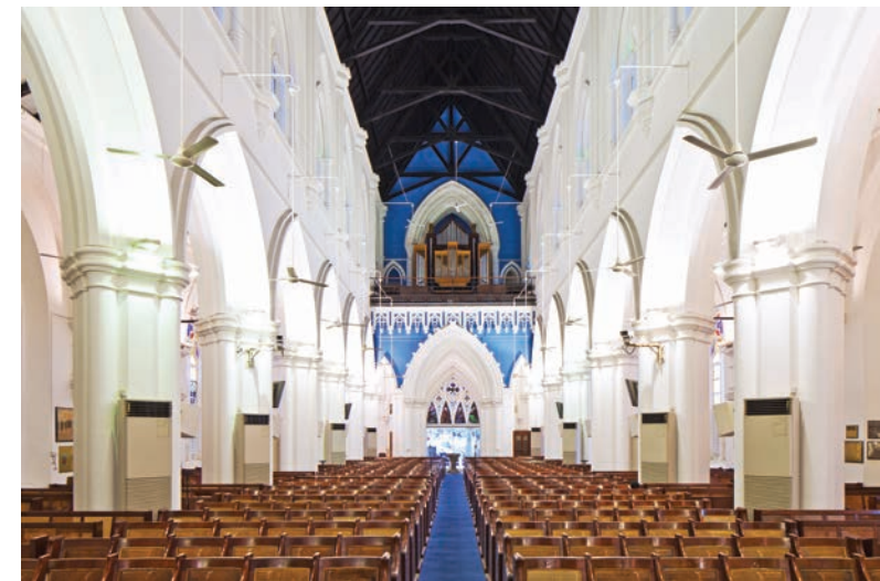
Air-conditioning units placed by the columns in Saint Andrew's Cathedral. Image courtesy of the Preservation of Sites and Monuments, National Heritage Board.
