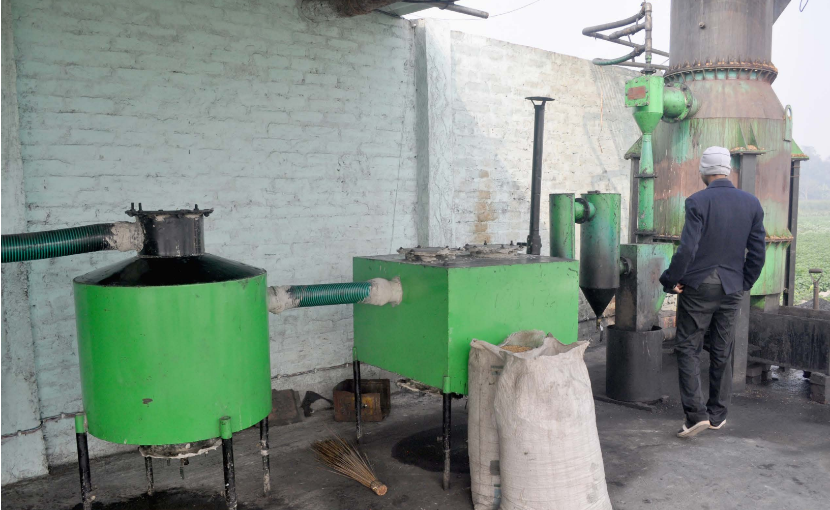
A biomass gasifier plant at a HPS microgrid site in Bihar, India
