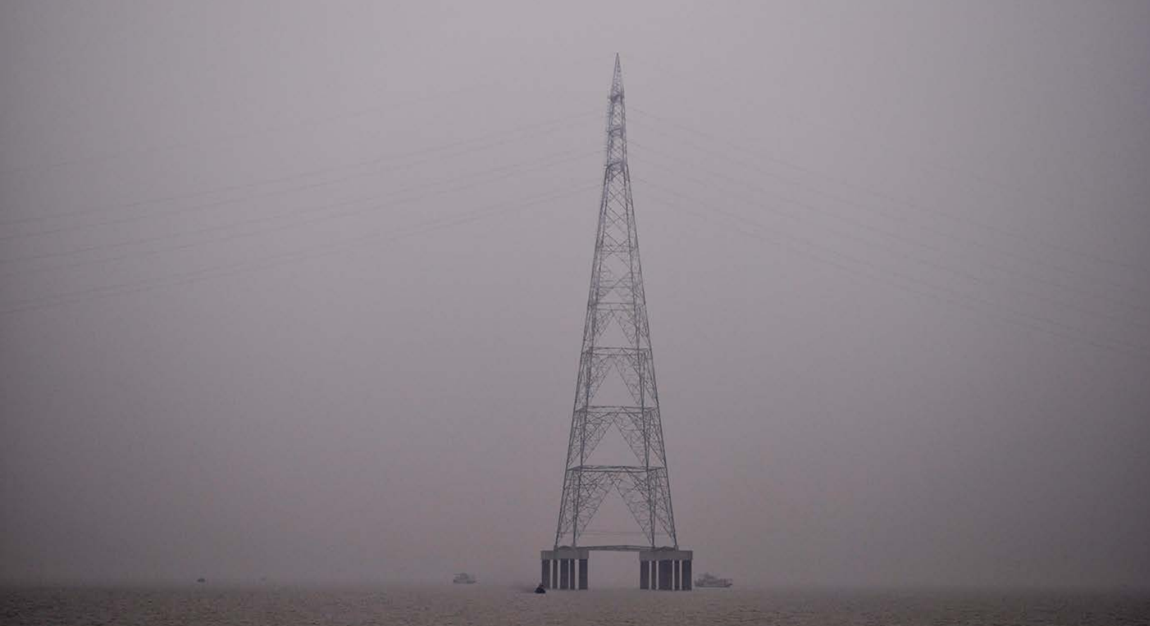
Off-shore transmission line connecting the Sundarbans Islands to the West Bengal central electric grid
