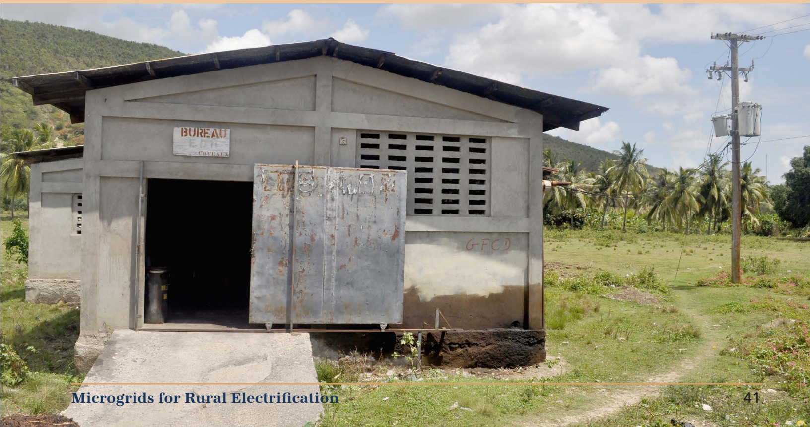
The generator house and step-up transformers at the Coteaux microgrid in Haiti
