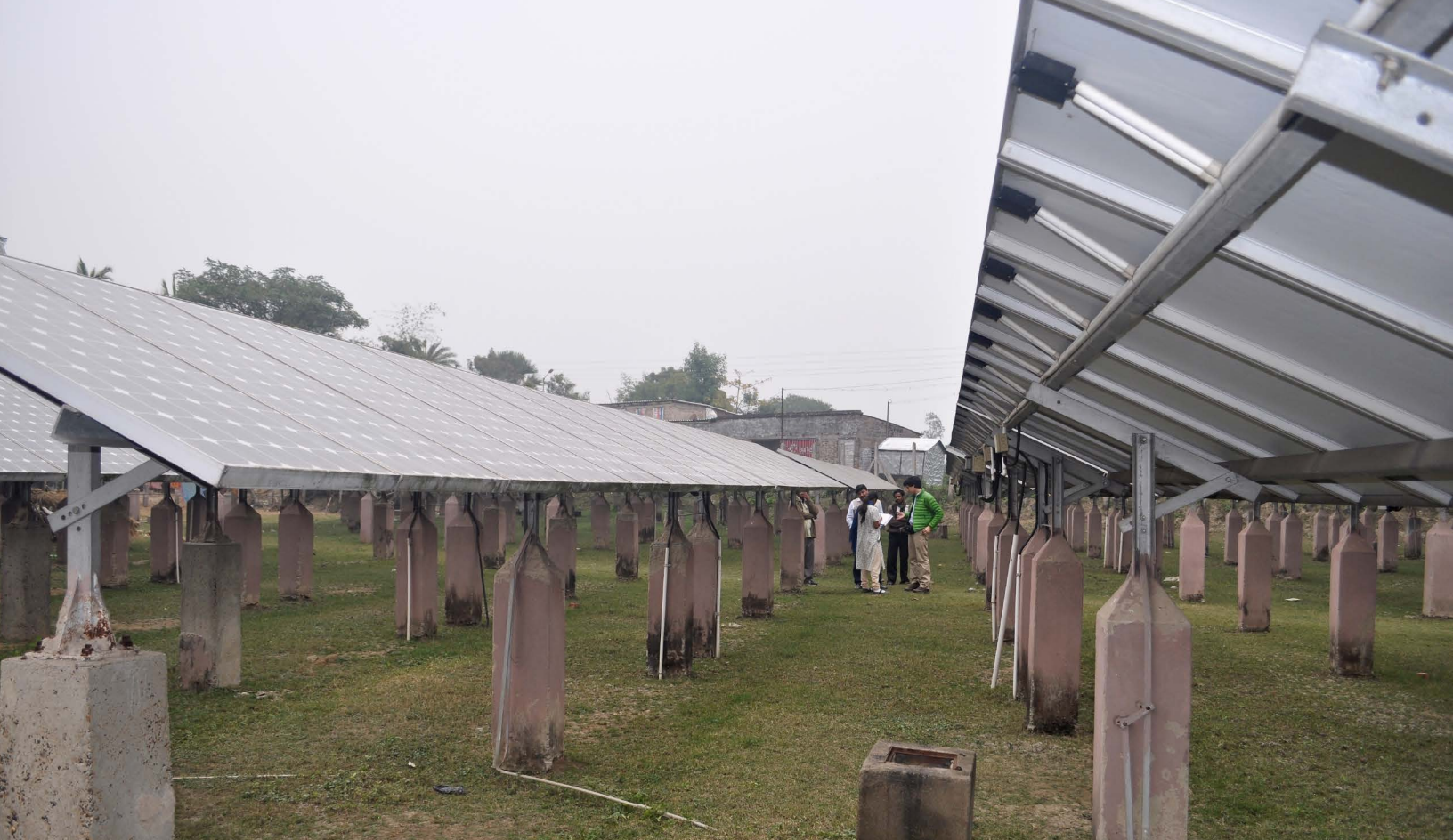
A glimpse of the 120 kWp solar PV array at a WBREDA microgrid site on Sagar Island, India
