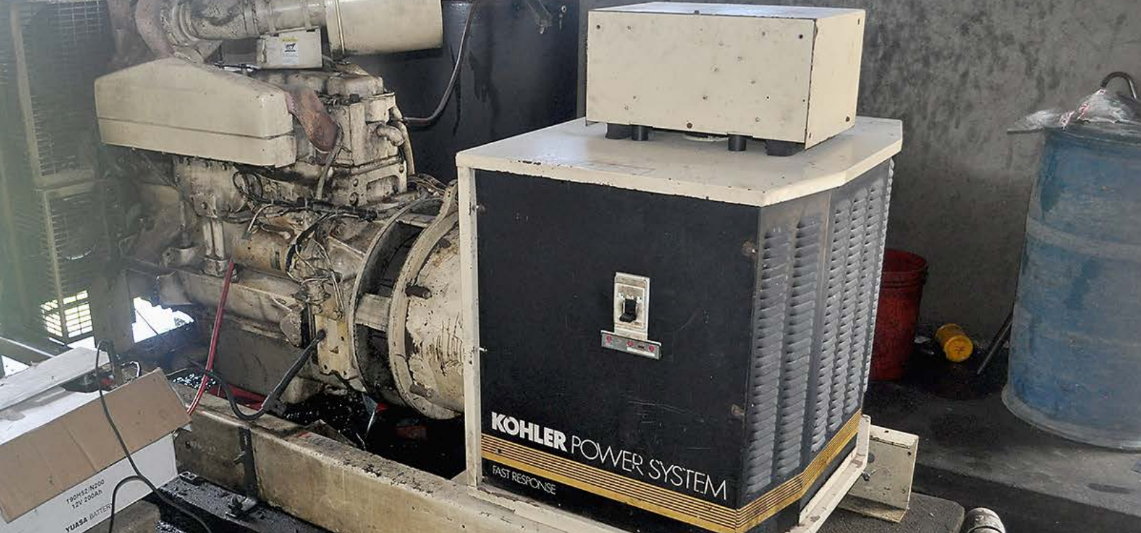
Diesel generator in need of repair that powers the Coteaux microgrid in Haiti, built in 1994
