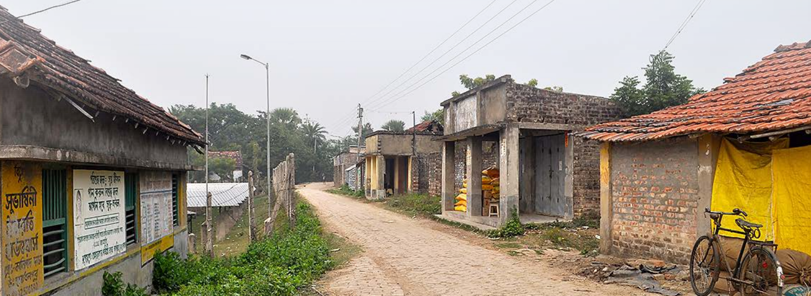
A street with distribution lines at a WBREDA microgrid site on Sagar Island, India.
