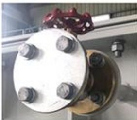
Oil Fill Valve
