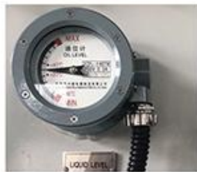
Liquid Level Indicator
