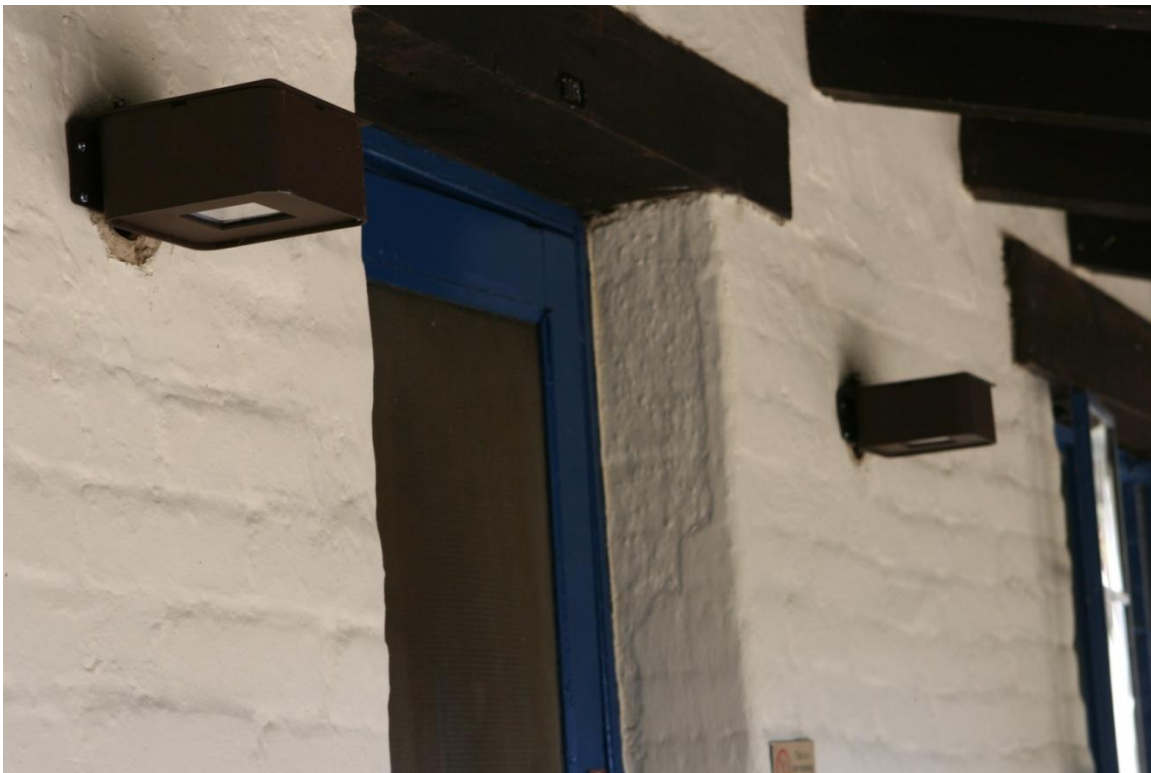
Figure 10. LED shoebox style used as wall mount building egress and patio lighting in Big Bend National Park.
