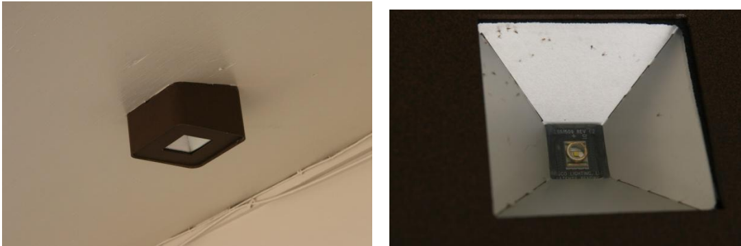
Figure 12 a-b. Under canopy fixture with wiring in soffit at Big Bend National Park, close-up shows deeply recessed single LED lamp.
