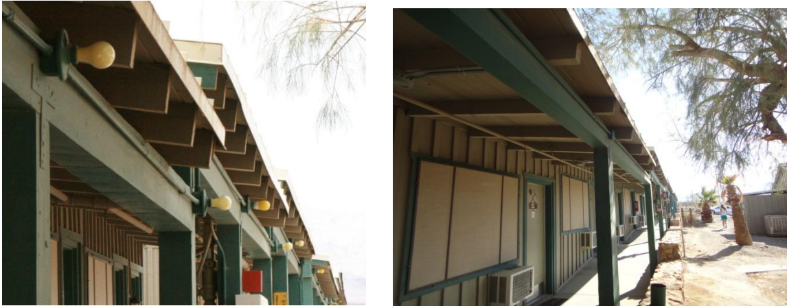
Figure 4a-b. Before/after: Unshielded bare bulbs were removed during retrofit at Stovepipe Wells.
