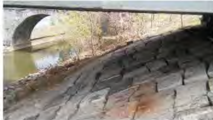
Limestone canal blocks placed under the southern Rexford Bridge abutment to prevent erosion. Remnant of the aqueduct visible in the background.
