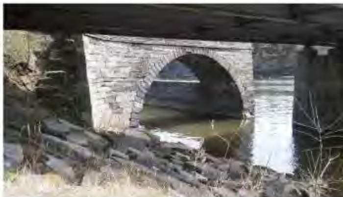
Canal blocks placed under the northern Rexford Bridge abutment. A section of the canal aqueduct is visible in the background.
