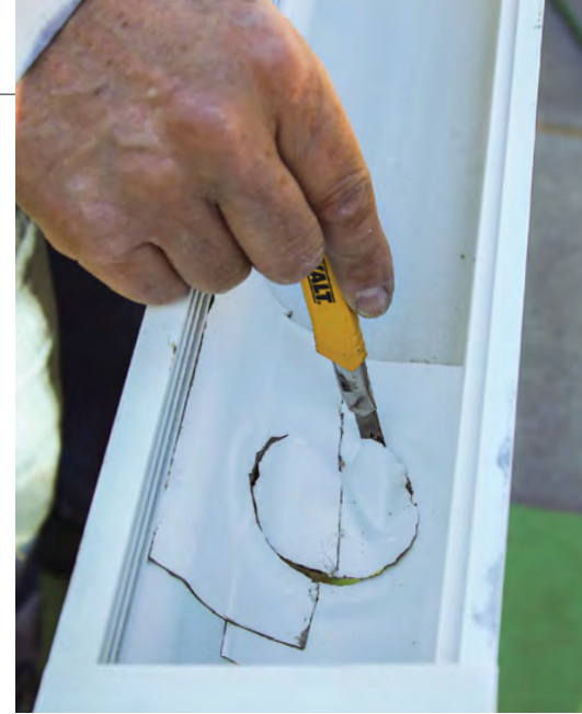
Make the opening. The top of the downspout outlet is sealed with pieces of butyl tape that are rolled with a small roller for a strong bond. Then the downspout opening is cut with a knife.
