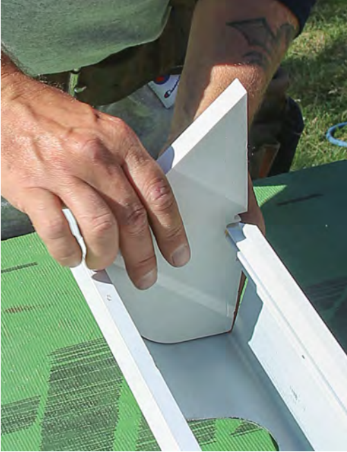
Install end dams. Plastic blocks are fit near rake transitions and sealed so water never reaches the mitered joint where the gutter meets the rake board. The blocks are angle-cut in the field to match the roof pitch.
