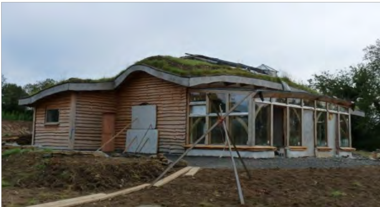
Lammas, Pembrokeshire: The community hub building is nearing completion and will be a focal point for the community and for events involving the local area. It is mainly built from locally sourced timber and stone, and incorporates renewable energy systems for electricity and heating.
