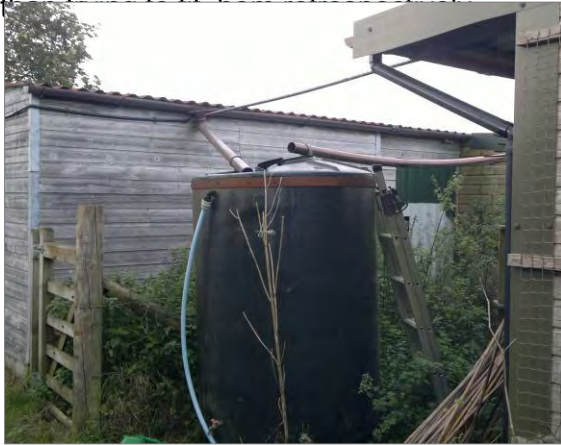
Water at Holsworthy Organics, Devon is collected from roofs and stored in containers above and below ground.
