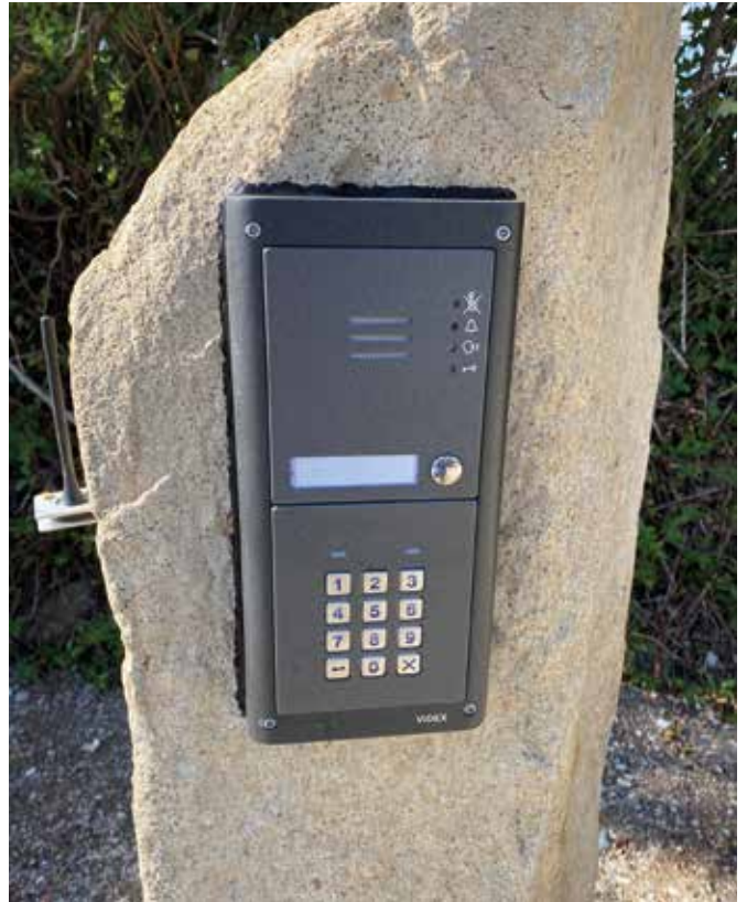
▲ Videx GSM Intercom with backlit keypad
