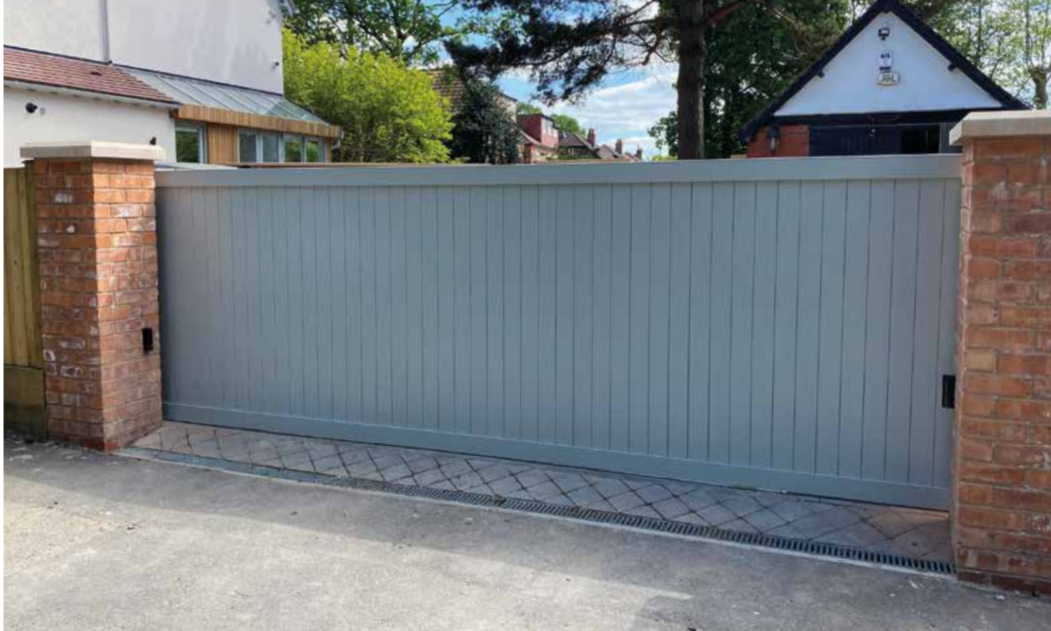
▲ Bottom tracked aluminium sliding gate, powder coated to match the new doors and windows.
