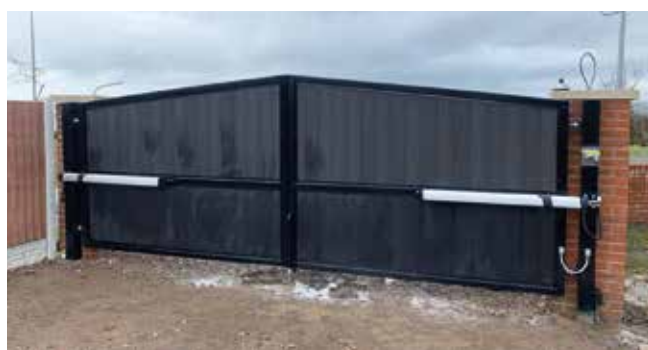
▲ Swing gates with above ground automation
