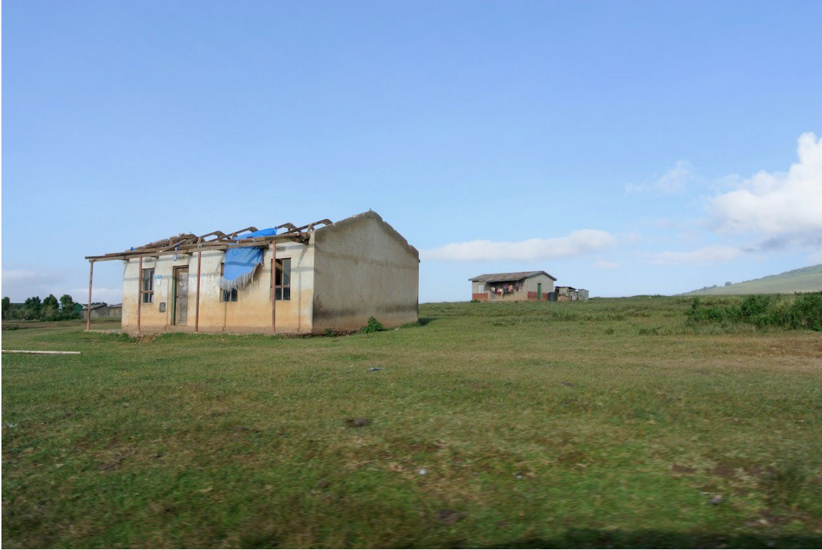
Mokilal village office, local government authority, with no roof in the Ngorongoro Conservation Area, Arusha region, Tanzania, on June 22, 2023. © 2023 Mathias Rittgerott/Rainforest Rescue
