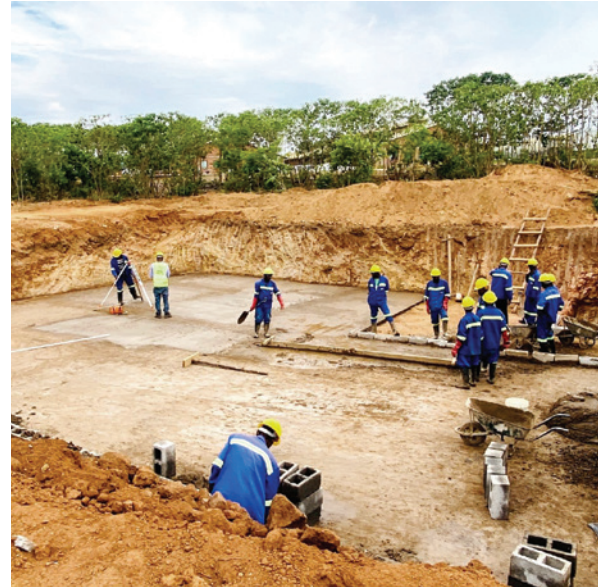
Construction of radiotherapy centre on-going in one of the first African countries to benefit from Rays of Hope support
