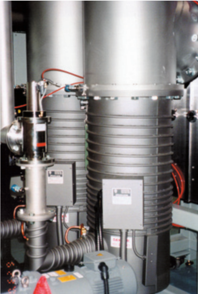
Courtesy of Mill Lane Engineering
