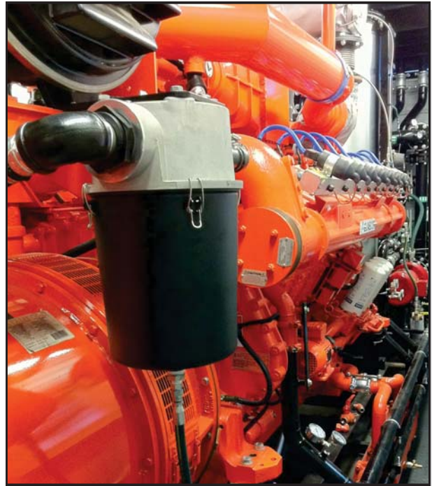
Closed Crankcase Ventilation System Guascor Engine Installation
