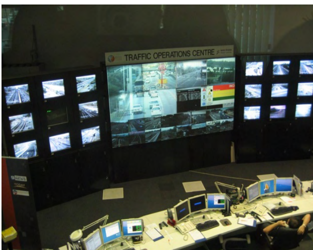
Main Roads Western Australia Traffic Operations Centre
