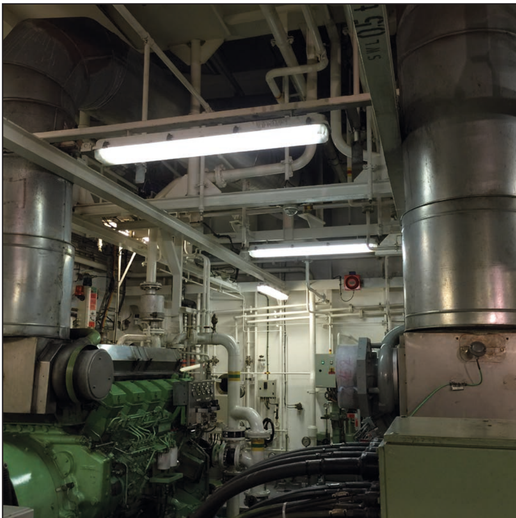
Figure 1: Location of the generator with the loose oil plug and the adjacent generator with the uninsulated section of the exhaust piping
