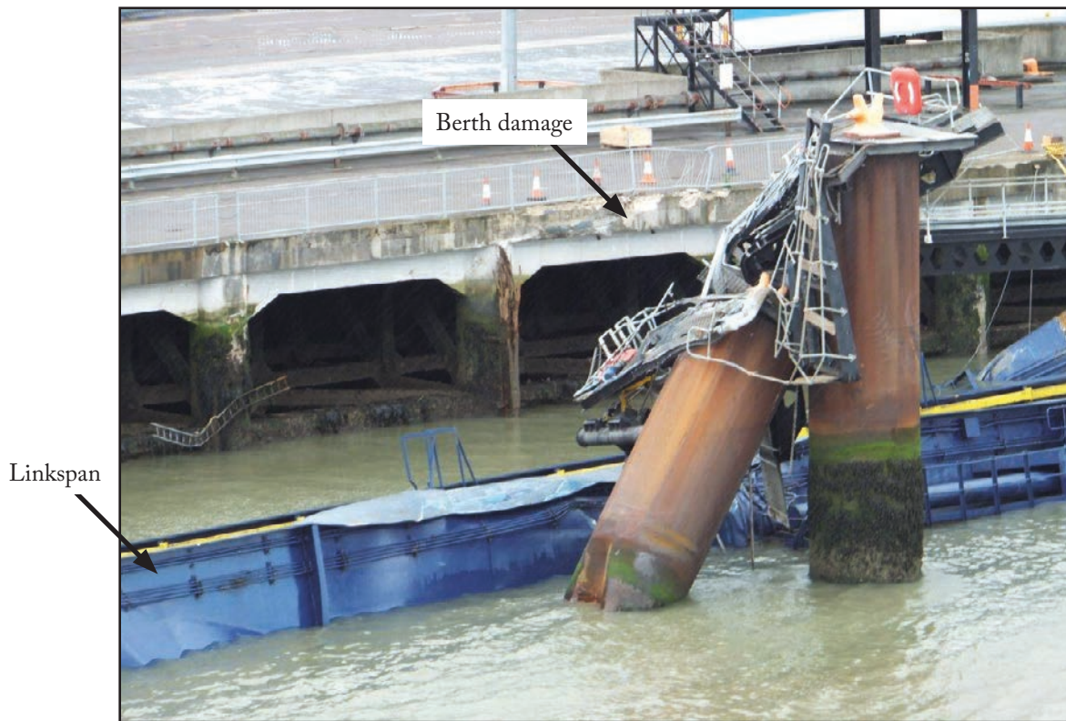
Figure 3: Damage to linkspan, mooring towers and berth
