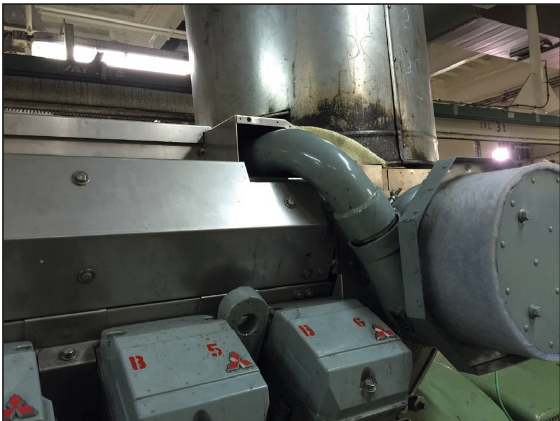
Figure 2b: Section of exhaust casing concealing the uninsulated section of exhaust piping
