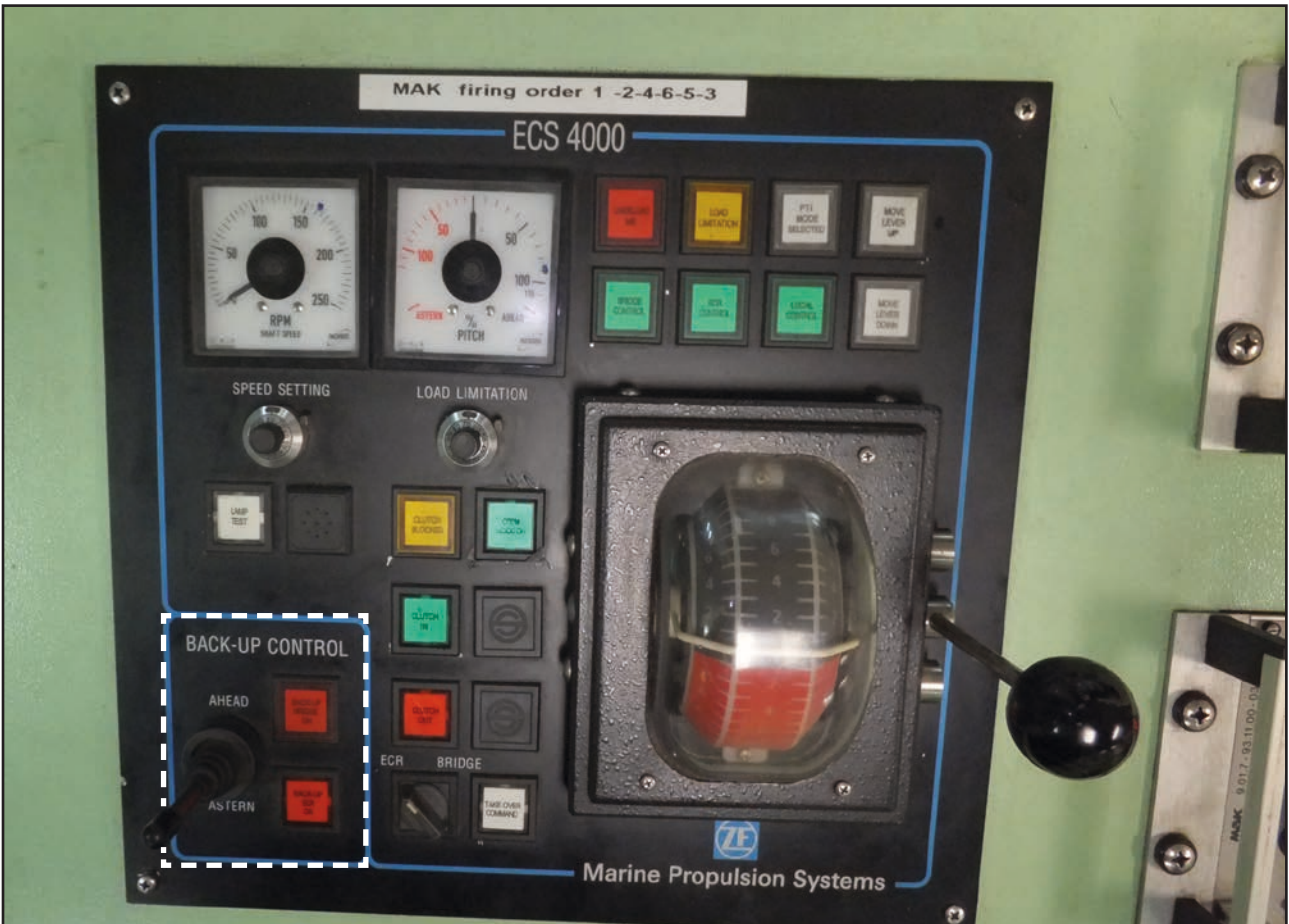
Figure 2: Bridge control panel of CPP system showing back-up controls
