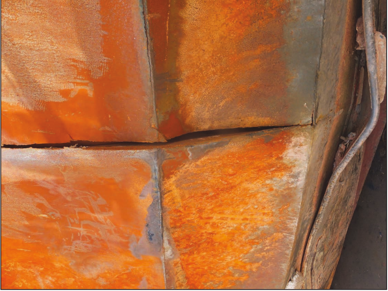
Figure 28: Split in welded joint in way of port side engine room/fish hold bulkhead
