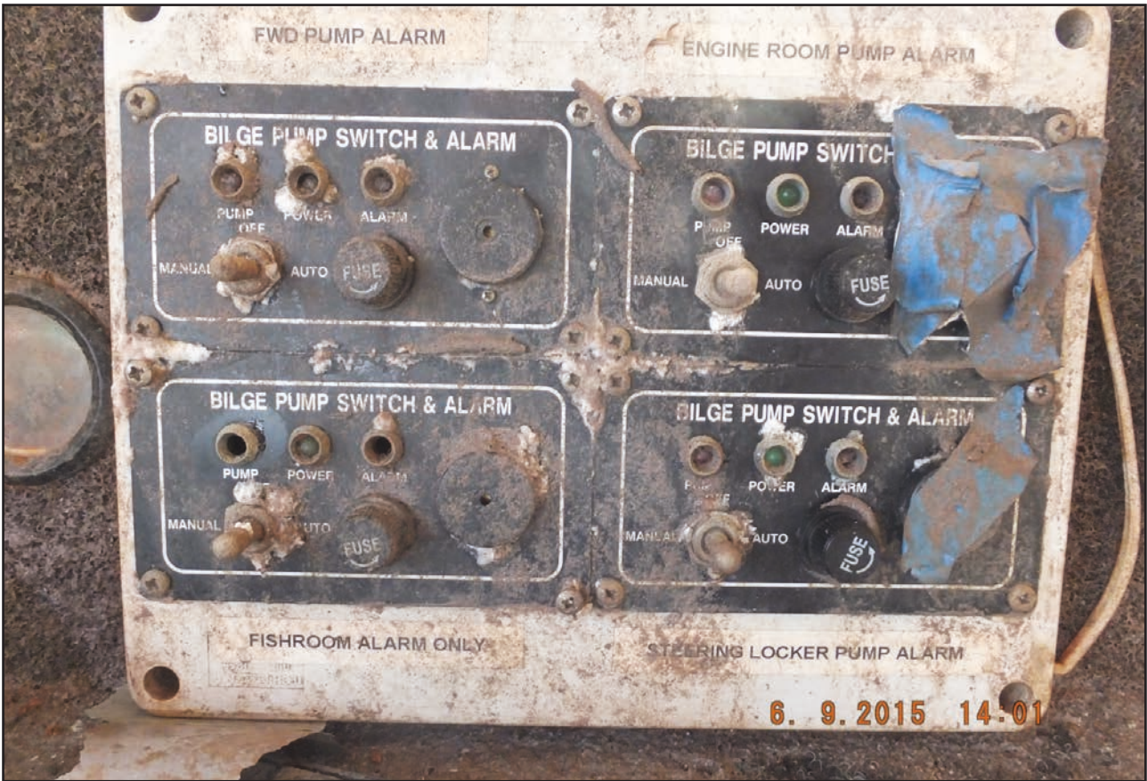
Figure 29: JMT's bilge pump switch panel
