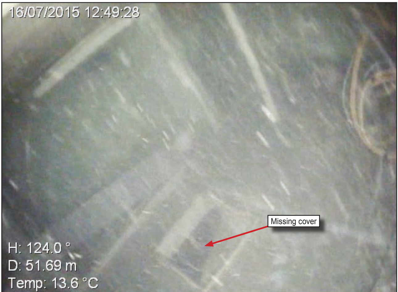
Figure 22: Missing shaft inspection hatch cover
