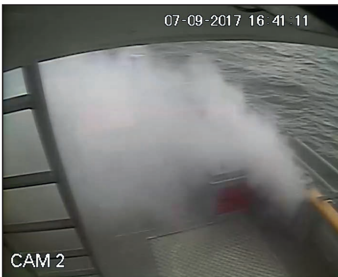
Figure 4c: Fire extinguishing powder billowing from the natural air vent
