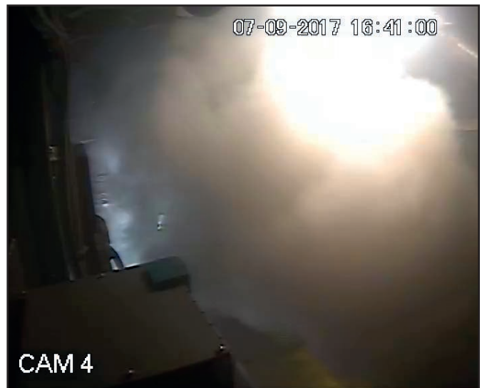
Figure 4b: Port engine space immediately following the operation of the fixed fire extinguishing system
