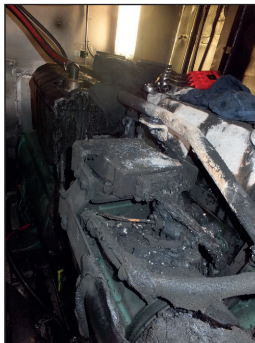
Figure 5b: Fire damage to port engine
