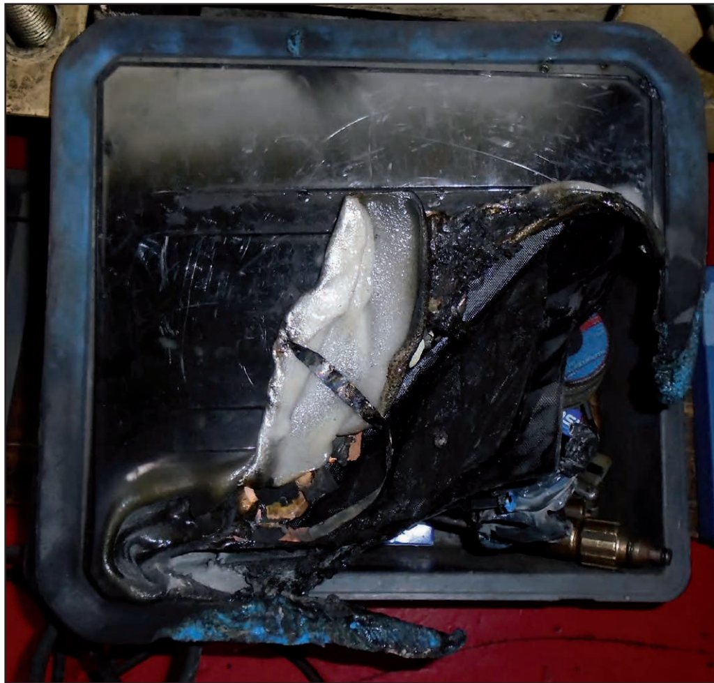
Figure 2: Damaged light unit
